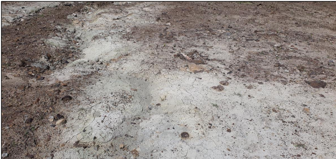
Figure 4-18: Problematic/unsuitable subgrade soil (Yellowish to whitish silty clay soil)
