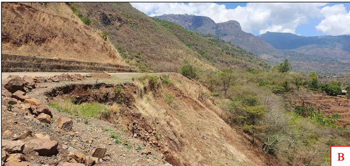
Figure 3-3: A) Visible significant cracks on the surface of fill slope B) Bulging & deformation on the surface of fill slope @ km 126+000 RHS
