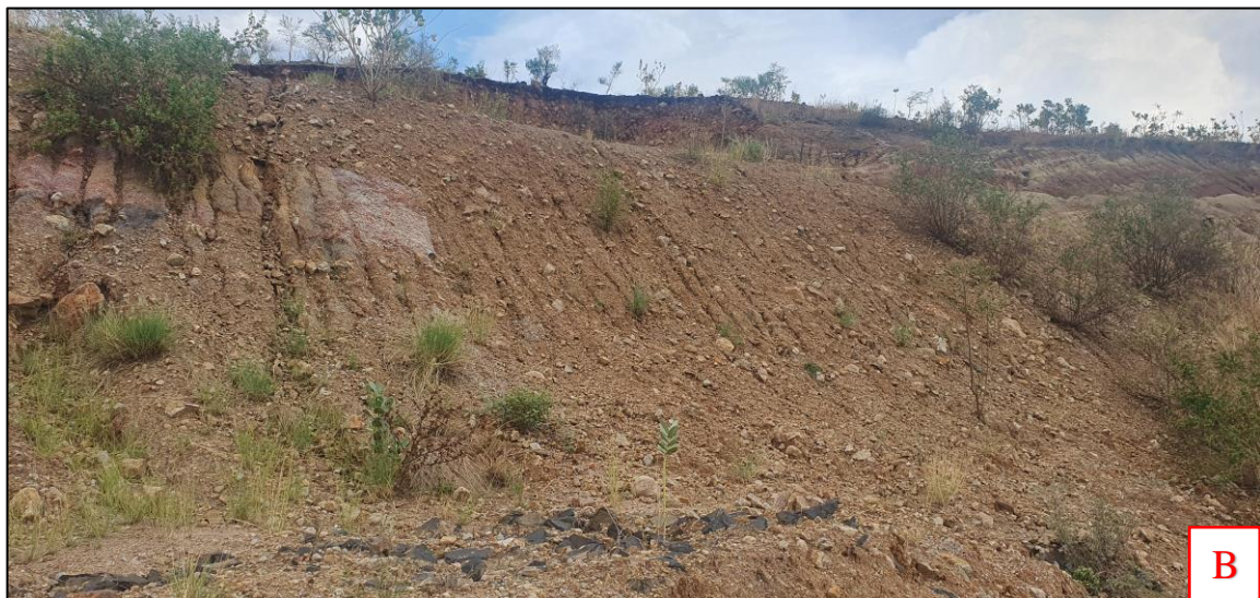
Figure 4-9: A) Exposed plant roots and vegetation loss on the surface of a slope B) Disappearance of grass, shrubs and trees due to erosion washing away the topsoil
