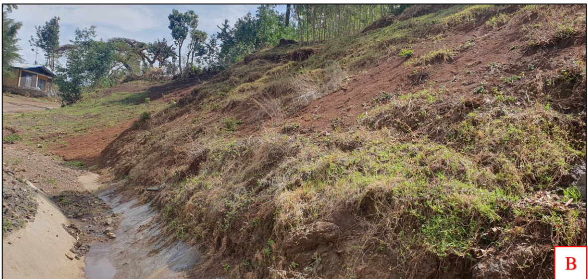
Figure 4-1: A) Wet patches exposed on the surface of a road cut B) Out flow and seeping of water from high ground in the pavement and side ditch
