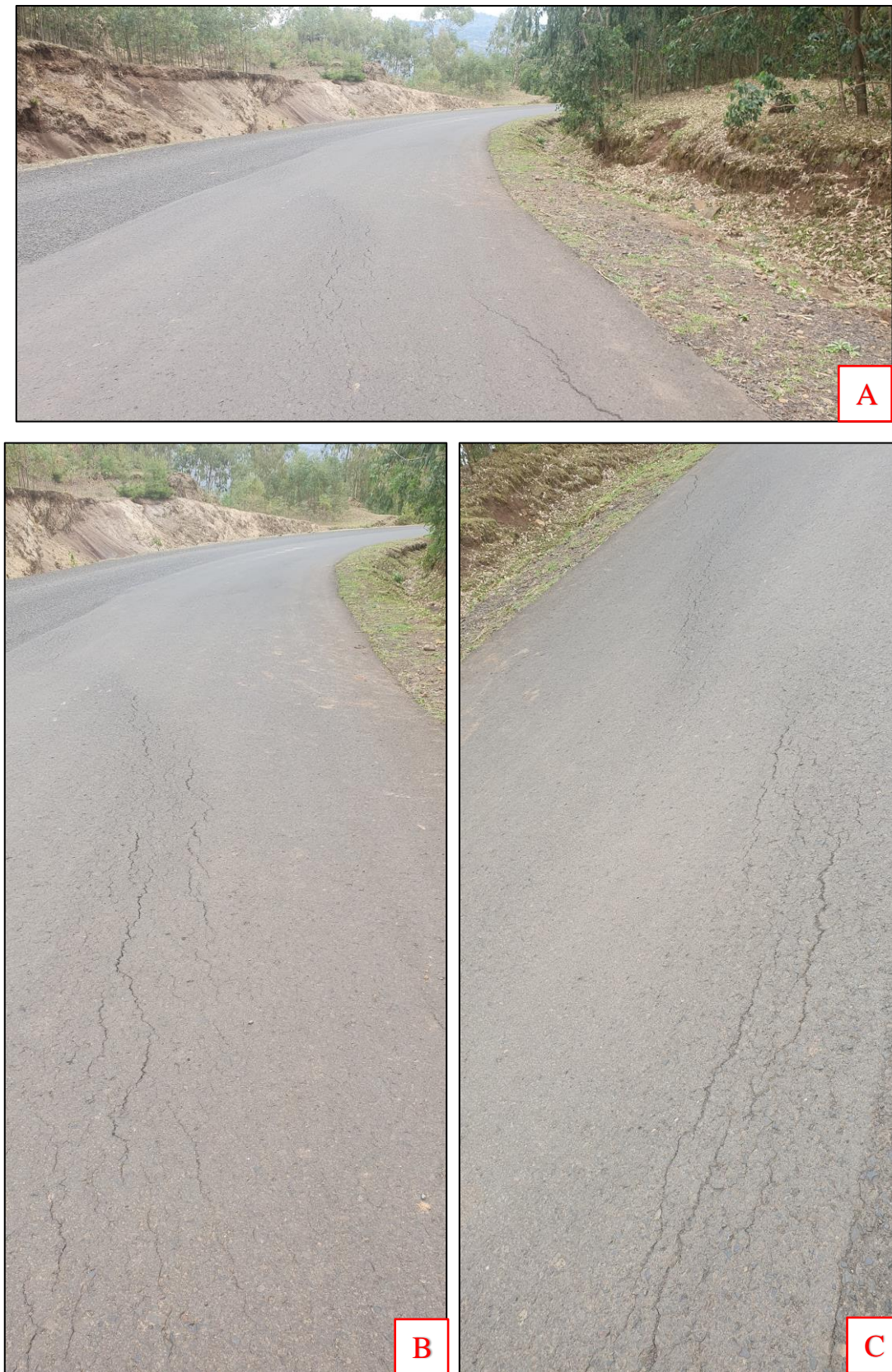
Figure 4-19: A) Surface undulation B) Surface cracking C) Settlement and depression
