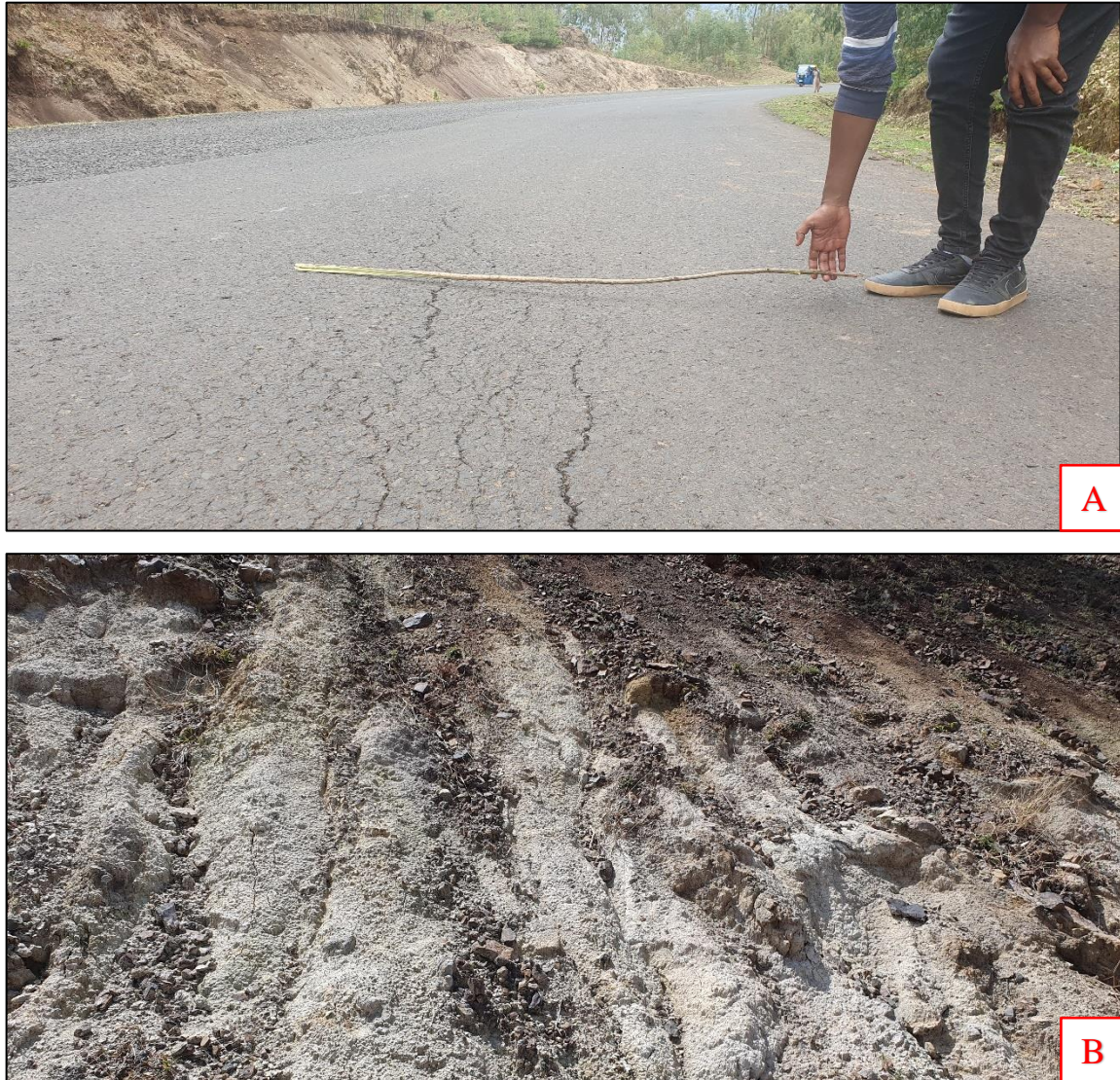
Figure 3-6: A) Cracks and uneven surface on newly placed asphalt B) Problematic/Unsuitable subgrade soil @ km 114+100 LHS
