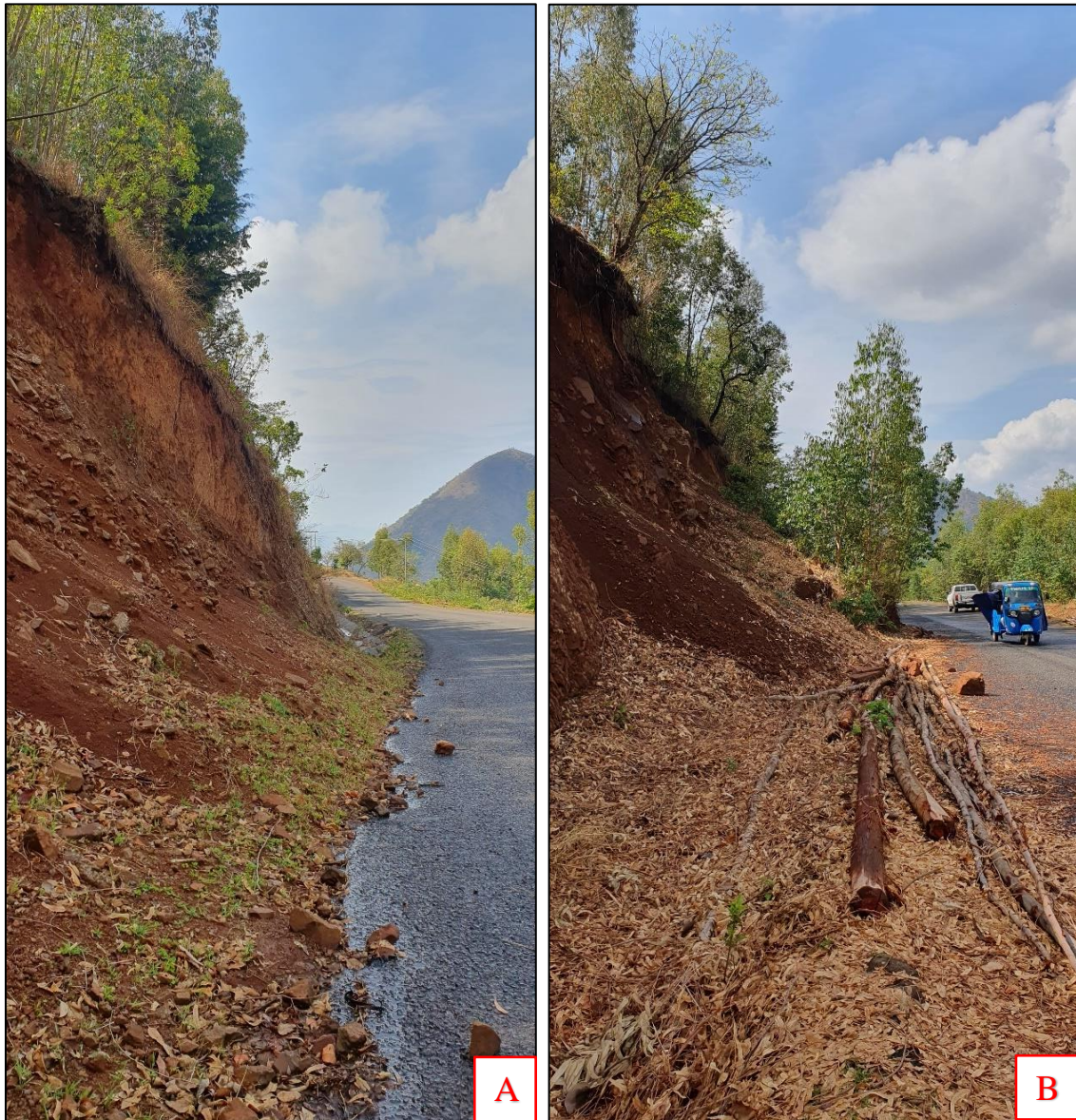
Figure 3-2: A) Slumping of soil mass B) Accumulation of displaced soil mass from the surface of cut slope @ km 100+300 RHS
