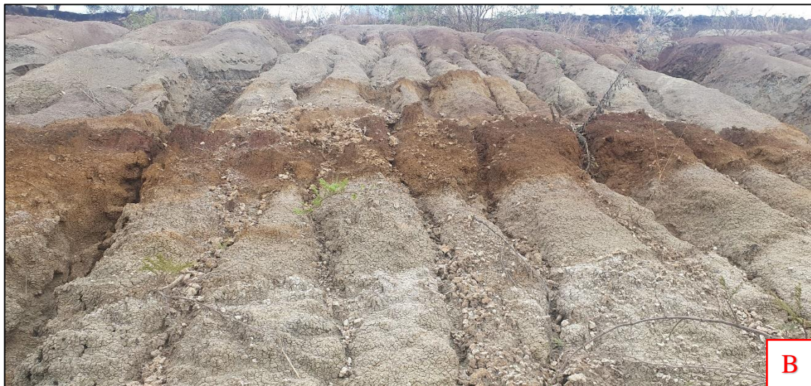
Figure 3-7: A) Accumulation of eroded soil in to the side ditch of the road B) Formation of gullies and channels on the surface of cut slope @ km 134+760 RHS
