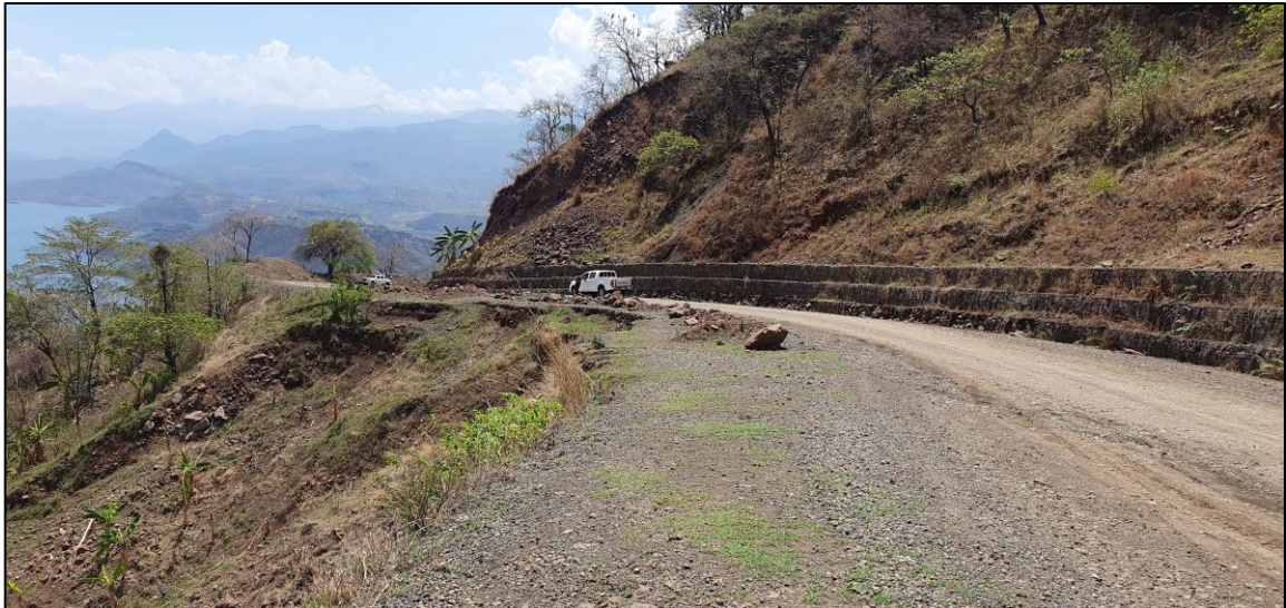
Figure 4-38: Significant signs of extensive cracking and settlements on the surface of road
