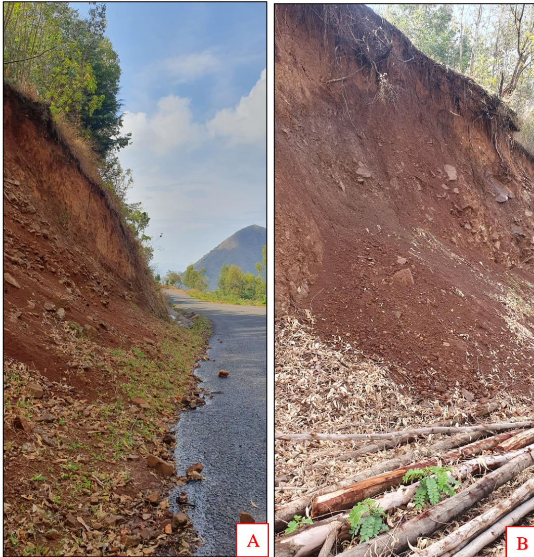
Figure 4-22: A) Slumping B) Accumulation of displaced soil from the surface of slope
