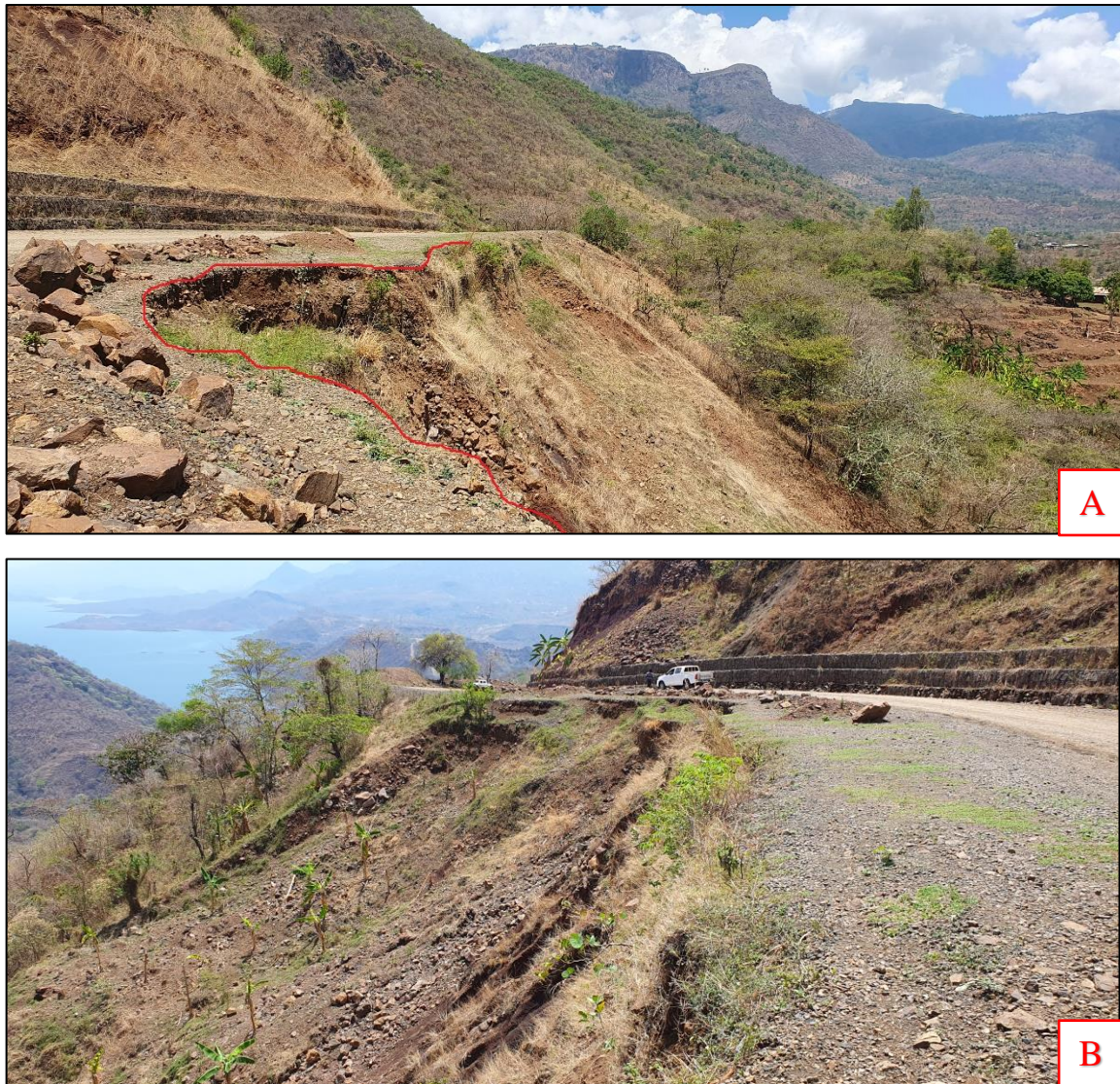
Figure 4-36: A) Visible cracks on the surface of roadside fill slope B) Bulging on the surface of fill slope
