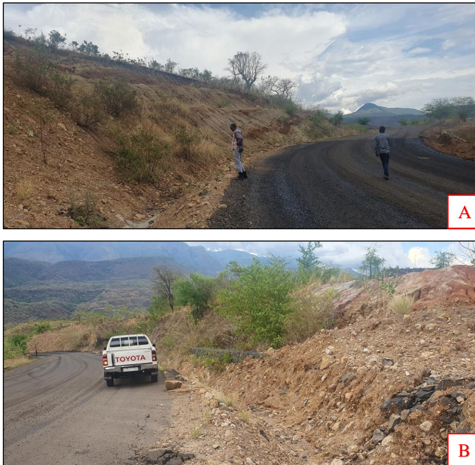
Figure 4-10: A) Accumulation of sediments B) Tilting of adjacent structure (gabion wall)
