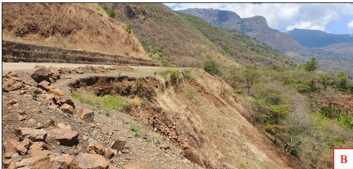
Figure 4-37: A) Deformations on the surface of fill slope B) Bulging on the surface of roadside fill slope
