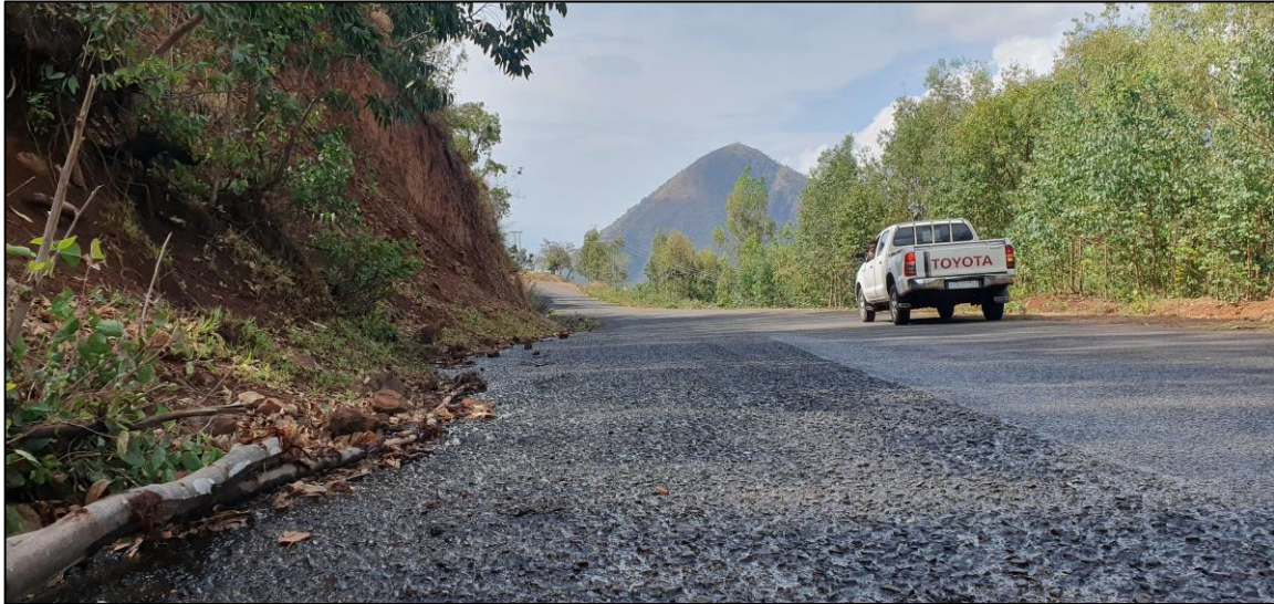
Figure 4-24: Debris flow near the toe of the failed slope @ km 100+300 RHS
