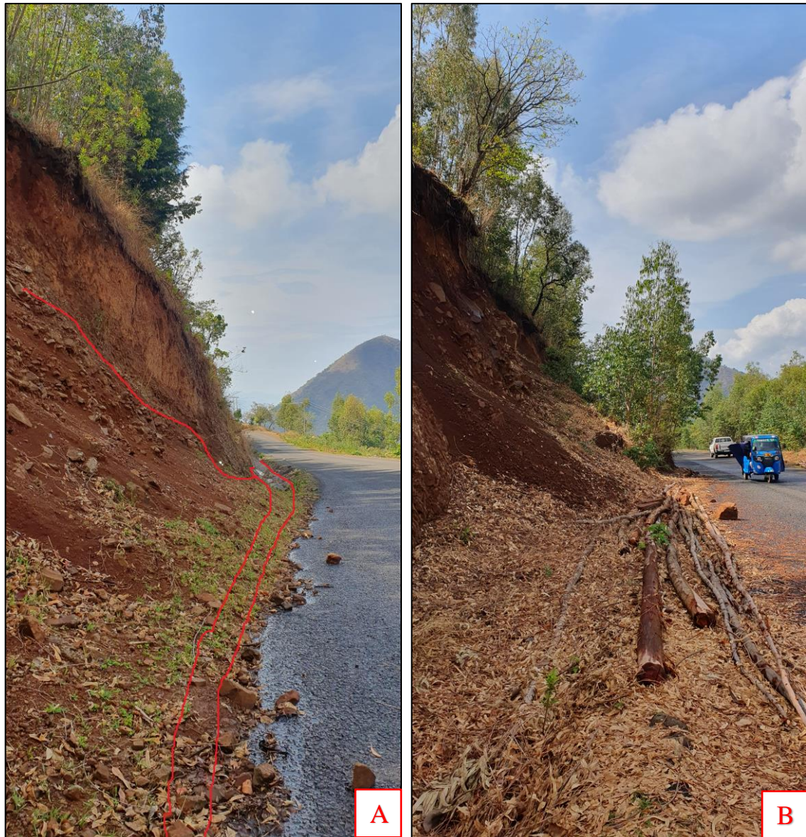
Figure 4-23: A) The side ditch adjacent to the road has been filled by sliding material B) A section of driving lane has been covered by the sliding material @ km 100+300 RHS
