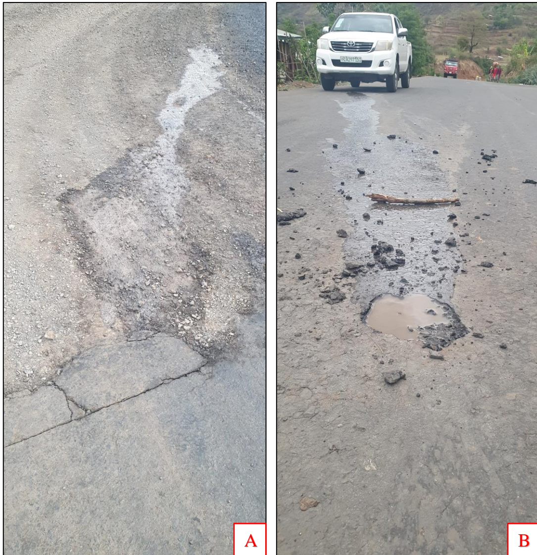
Figure 4-4: A) Road surface pre-mature failures B) Pumping out of water on the surface of the pavement
