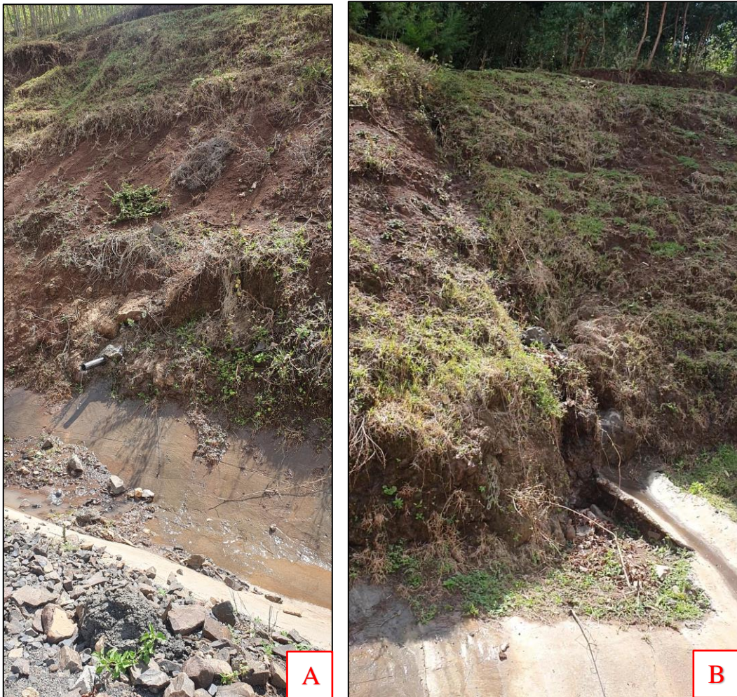
Figure 4-2: A) Visible outflows on the side of road cut B) Presence of hydrophilic vegetation on the surface of high ground
