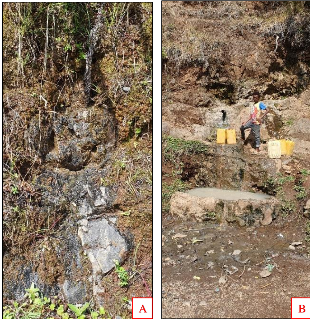
Figure 3-5: A) Wet patches at the surface of back slope B) Visible outflows from high ground to the pavement @ Km 105+000 RHS
