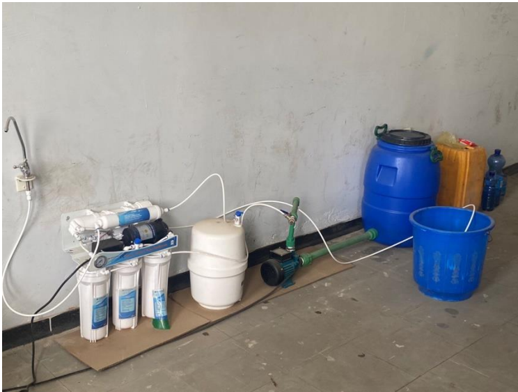
Annex 3: RO Filtration system setup
