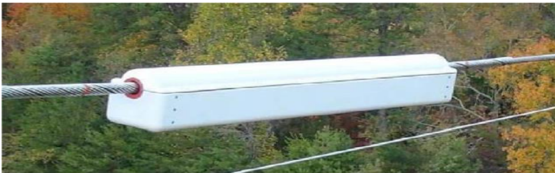
Figure 2- 4 DSR connected to a transmission line [10]
