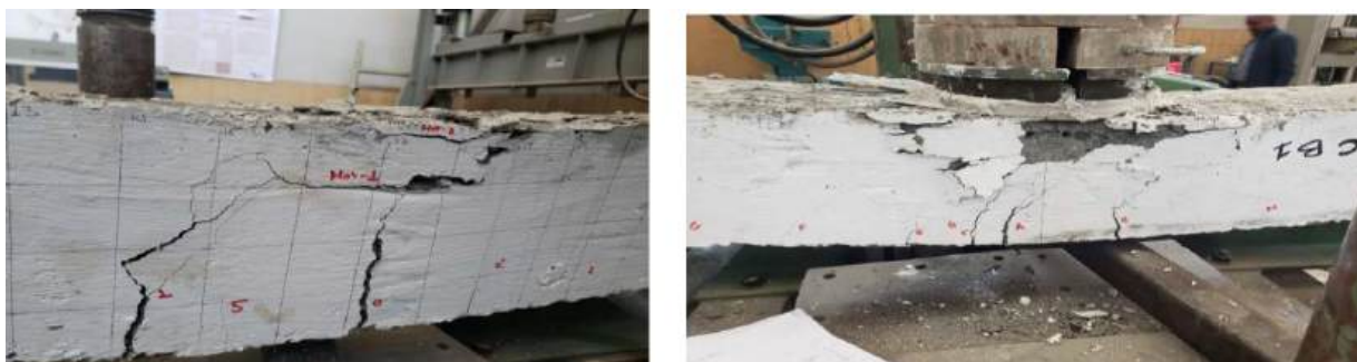
Figure 4.4: Flexural failure of G3B-30
