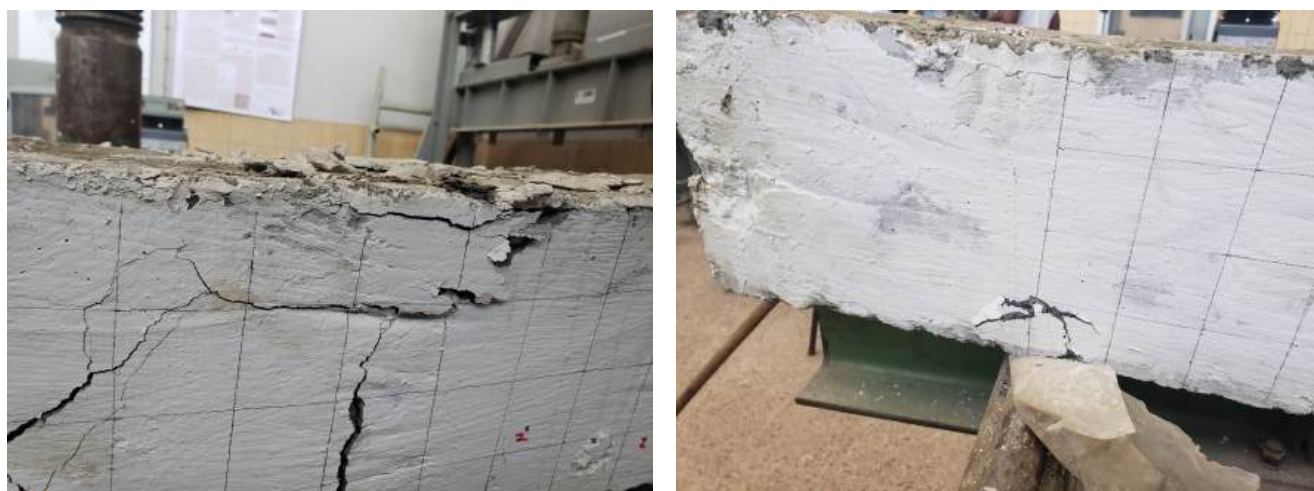
Figure A.15: G3B-30 Flexural Crack and Concrete Crushing at Mid Span & at Support
