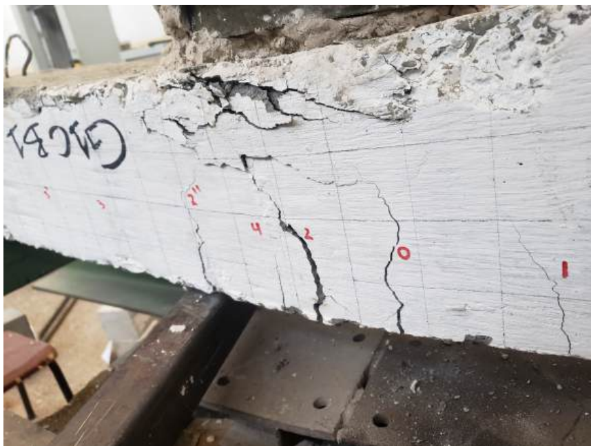
Figure A.2: Close up on the Failure State of G2B-20
