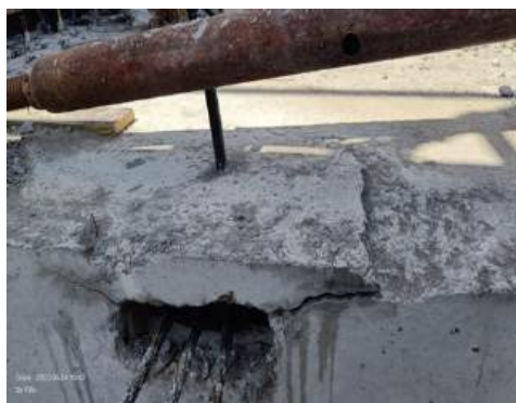
Figure 1.1: Instance of Anchorage Zone Failure
