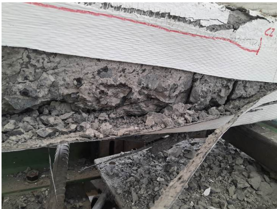
Figure A.23: Concrete Crushing and Spalling at Bottom of the Beam G3B-22
