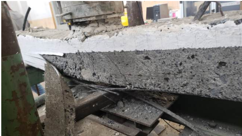
Figure A.19: G3B-21 After Failure
