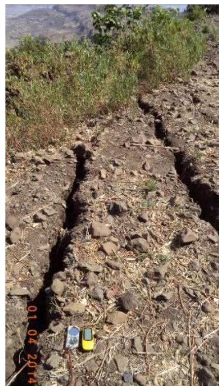
Plate 6.21 Deep vertical tension cracks observed after disposal material is damped on the slope
