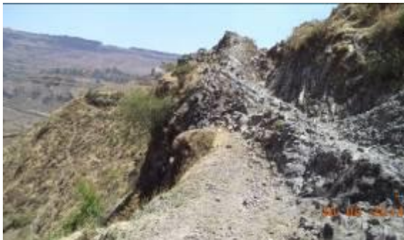
Plate 6.13 Photo showing loosening by opening of tension cracks in upper part of the slope
