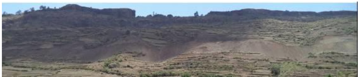
Plate 6.10 (c) Part of road under construction affected by rotational soil slide
