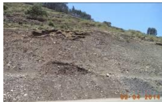
Plate 6.10 (a) Rotational slide in cut soil slope
