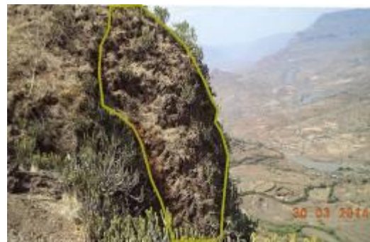
Plate 6.6 Photo showing rock block susceptible to fall or topple
