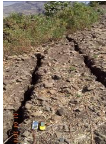
Fig 4.7b. Surface cracks observed on colluvial soil with strike in N - S direction.
