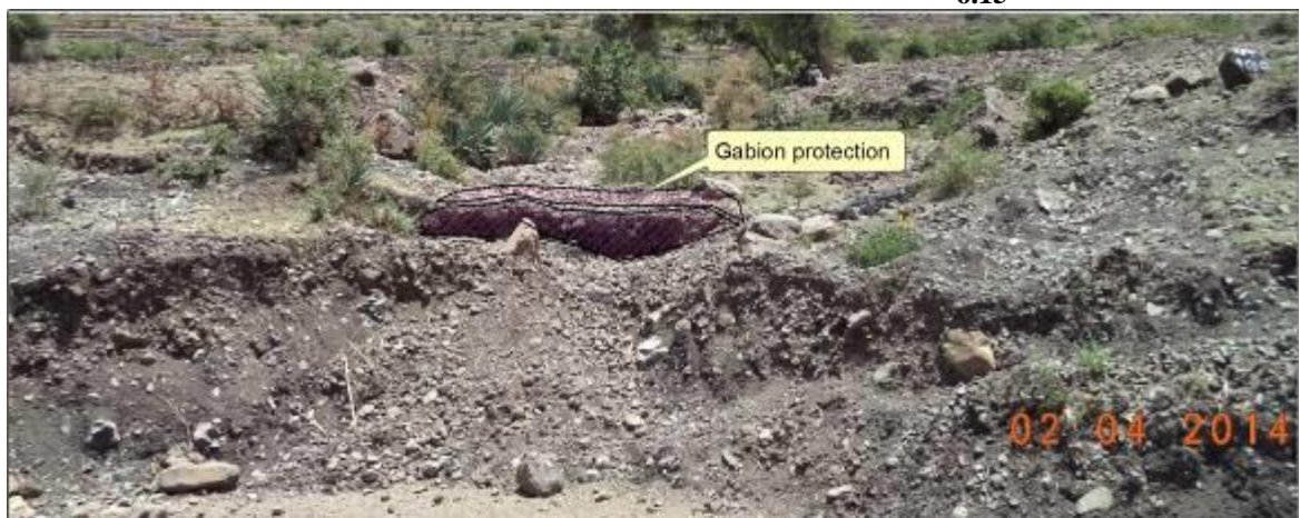
Plate 6.17 One of the gabion protections observed as manifestations of presence of slope instability in the area
