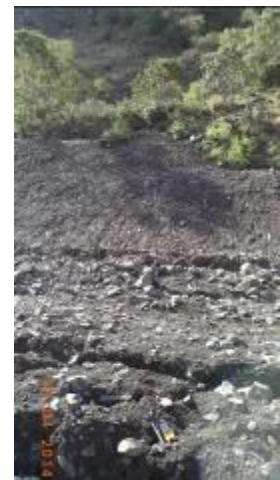
Fig 4.5c. Surface cracks on colluvial deposits at road cut section.
