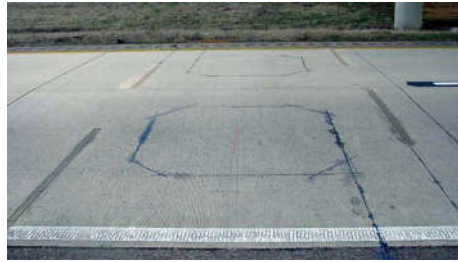
Figure 4-3: High-Speed WIM systems embedded in the pavement
