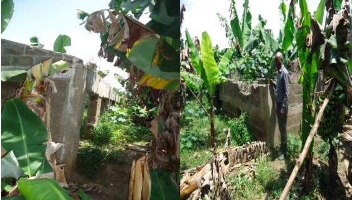
Figure 17: School building damaged by flood
