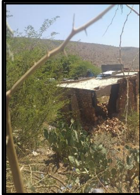
Figure 19. Series of cracks and collapse in buildings
