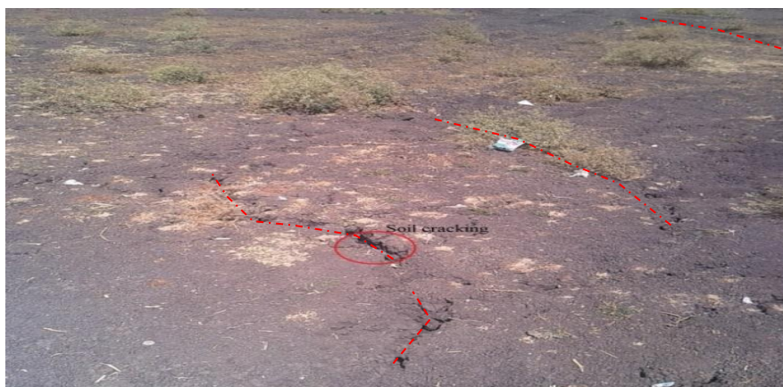
Figure 2.2: Photo taken from the site, where the black cotton soil showing visible cracks (red dotted lines).
