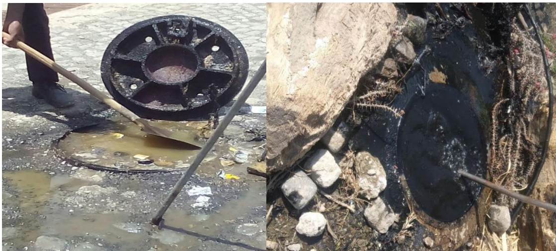
Figure 3:15 Photos of existing condition on the sewer network
