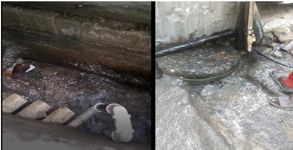
Figure 3: 12 Photos of illegal connection on the existing sewer network
