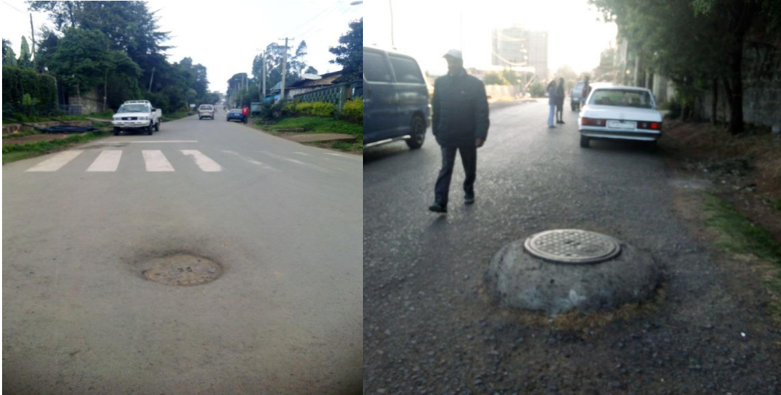
Figure 3: 14 Photos of Raised/Depressed Manhole covers on the existing sewer network
