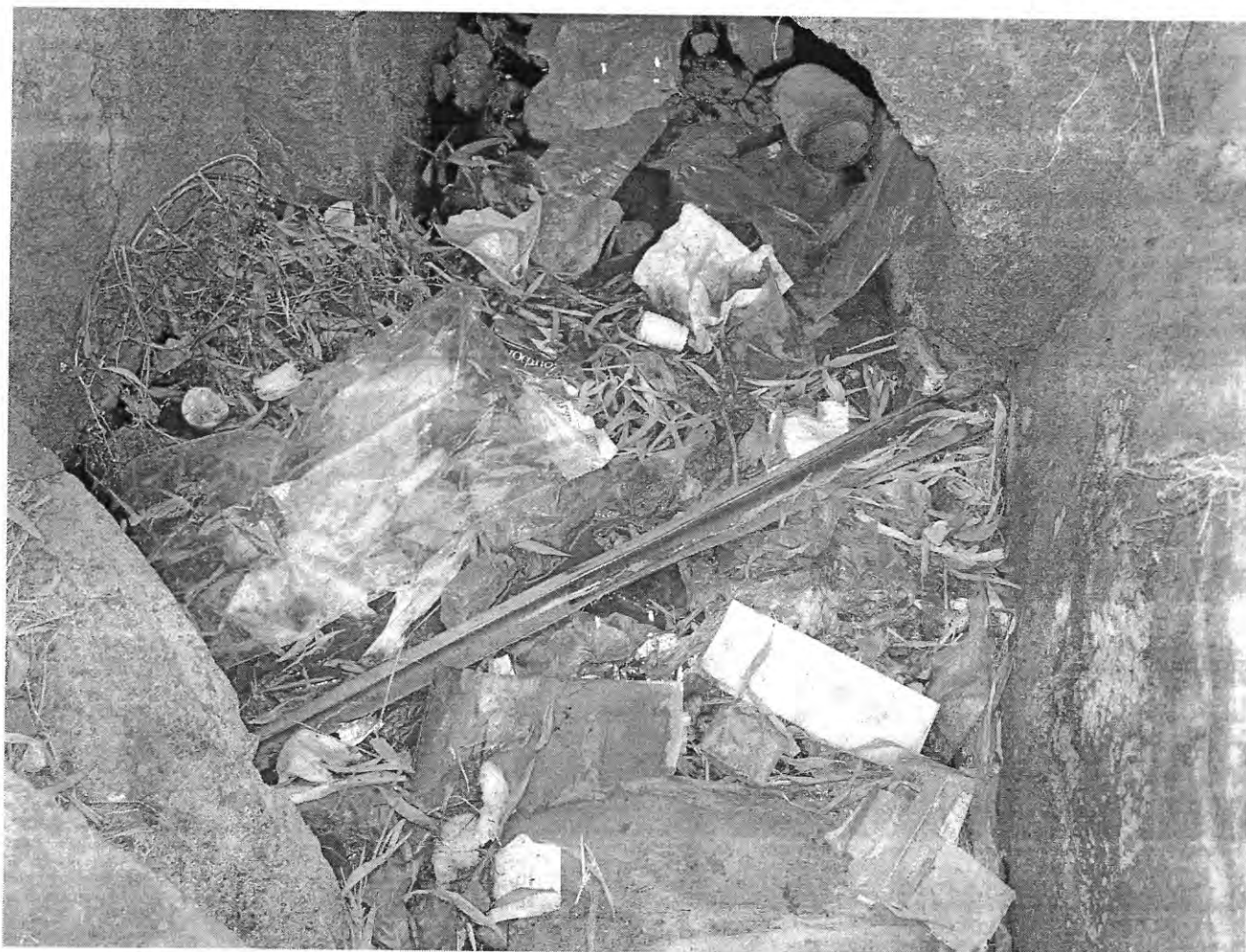
Picture 3.1 Drainage clogged with plastic bags waste Kolefe-Keraneo, Kebele 13/14
