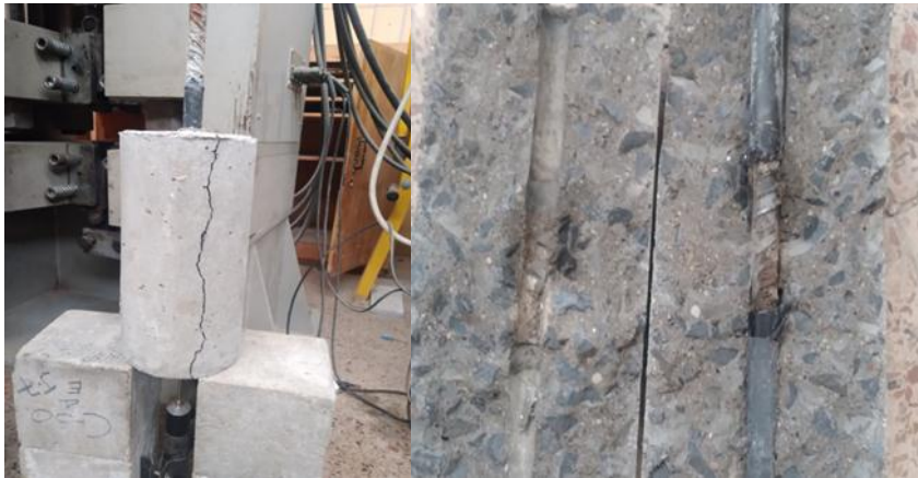
Splitting Bond failure
