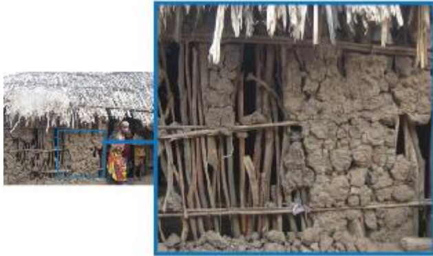
Figure 24- Inconsistency and lack of surface formation in traditional earthen construction, Bisidimo village. Source; the peace traveler.
