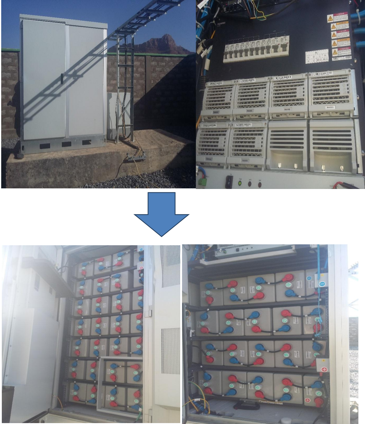
Figure 3: Battery bank used in the site
