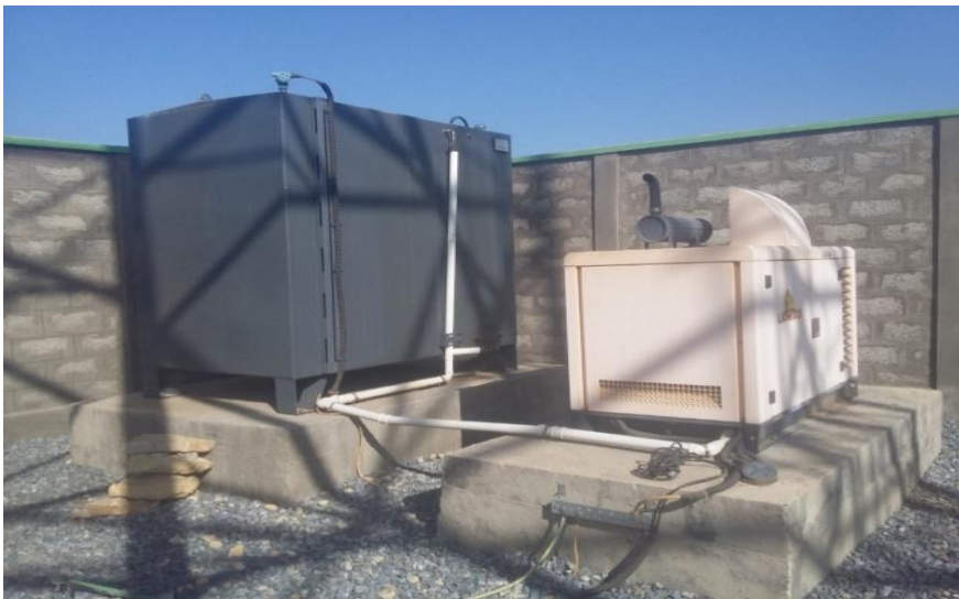
Figure 2: Generator plus fuel tank used in the site
