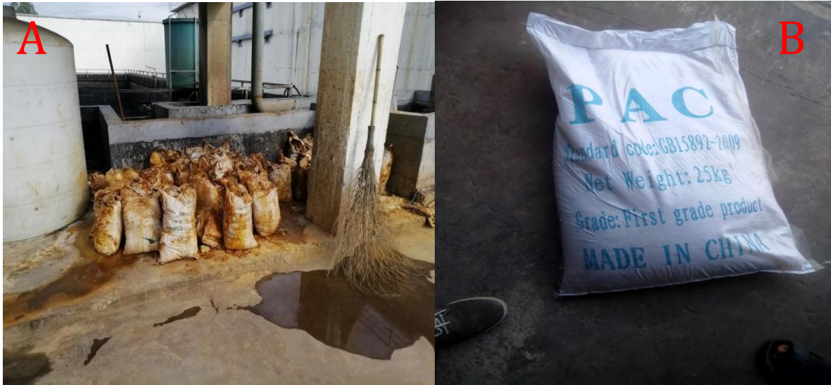
Figure 4.6: the expired chemicals (A) and (B) chemical that has treatment plant
