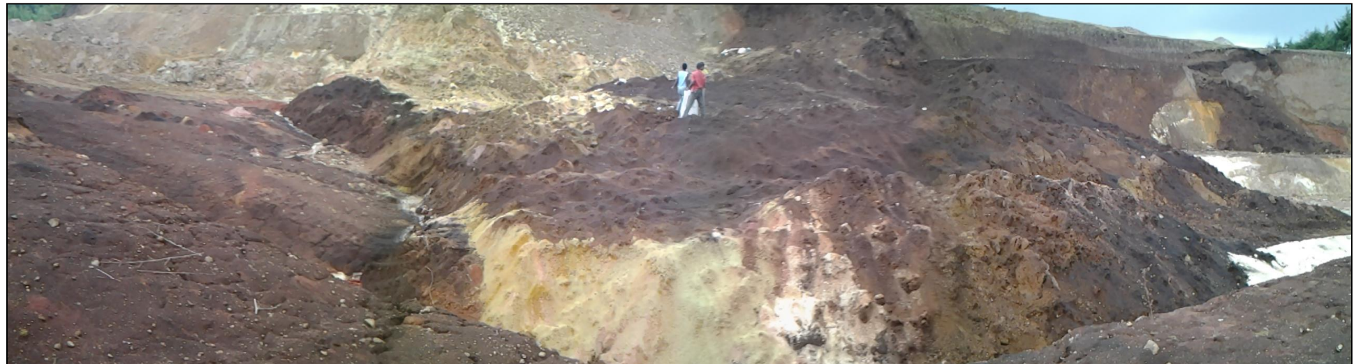
Figure 4.32: Displaced material at foot of the cut slope slide from Sta. 72+740 to Sta.72+790 LHS: front view
