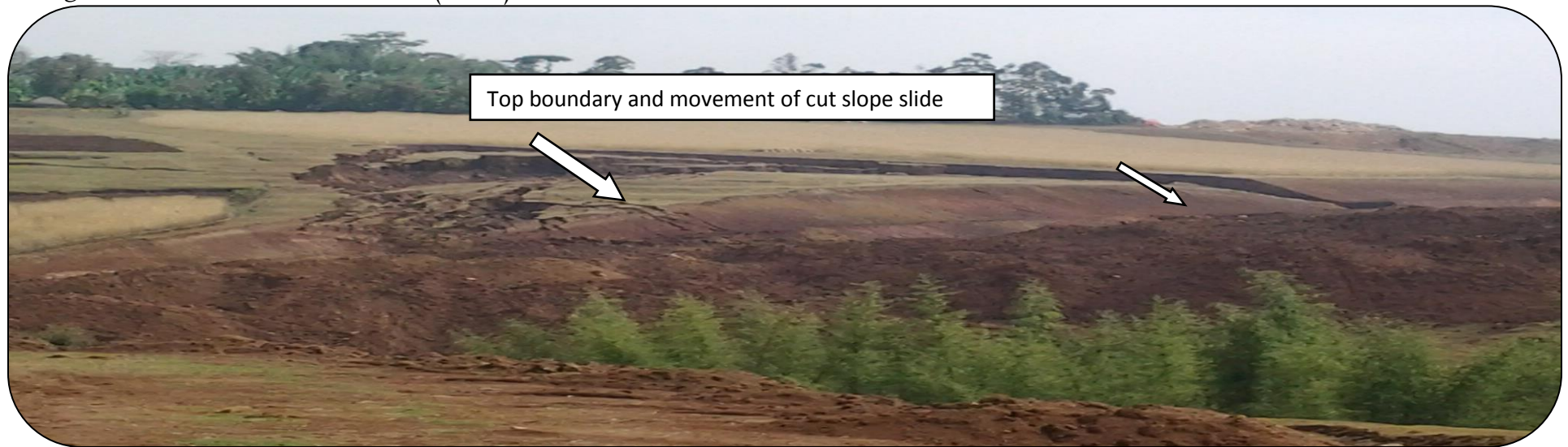
Figure 4.20: Slide manifestation from 68+020(Ahead) to 68+140(Back) RHS
