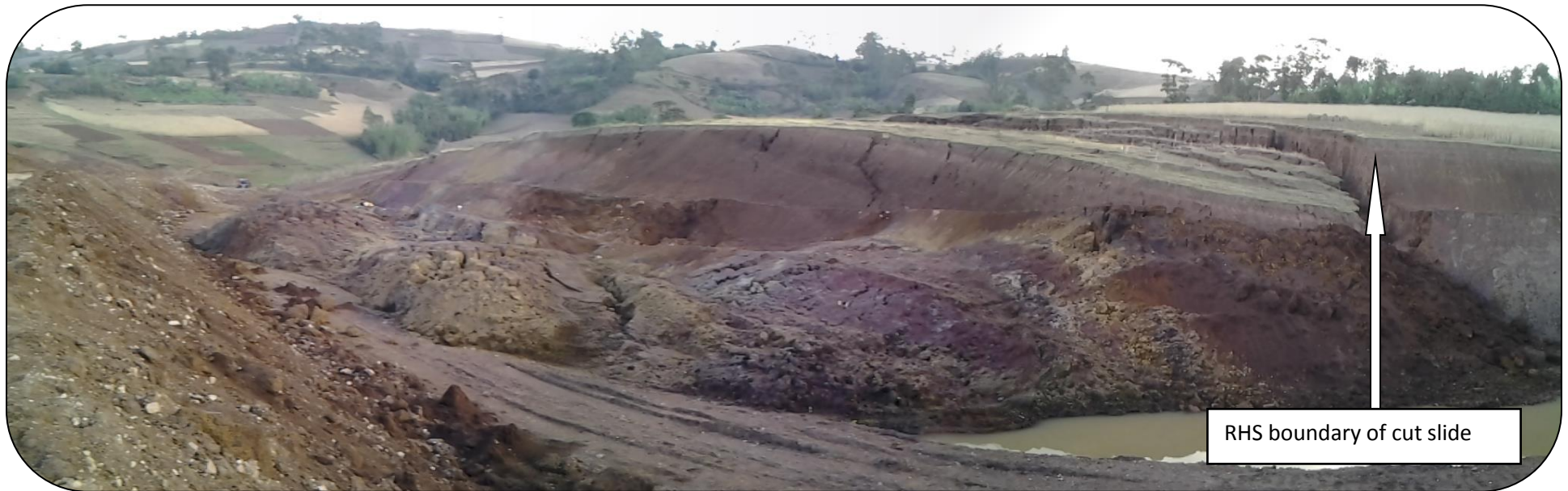
Figure 4.19: Slide at Start of Sta.68+020(Ahead)
