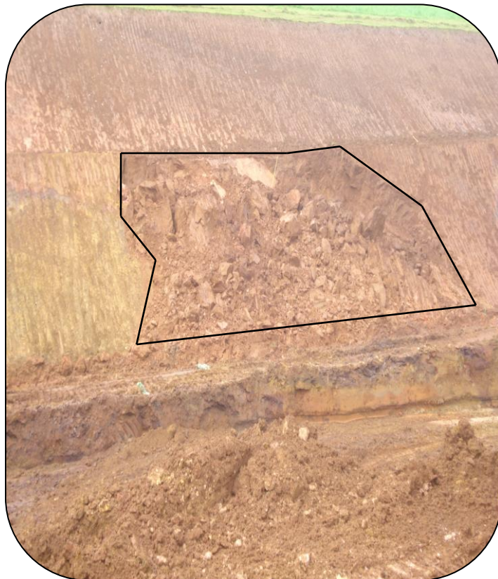
Figure 4.14: Initial Wedge Slide day lighting on the slope during progress of excavation work
