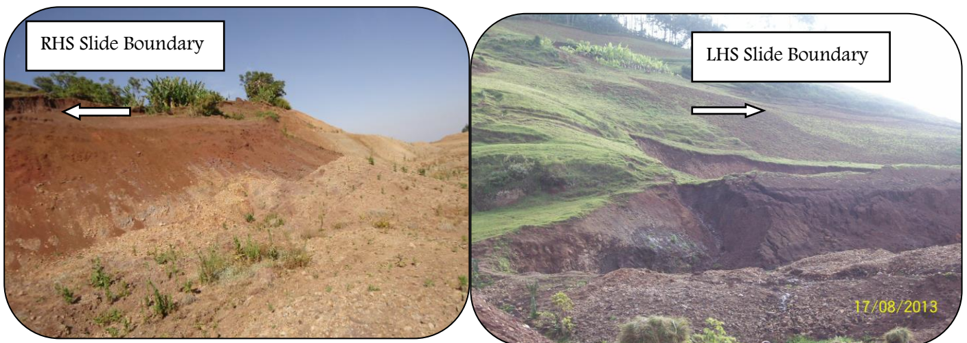
Figure 4.4: View of the failed cut slope RHS and LHS boundary
