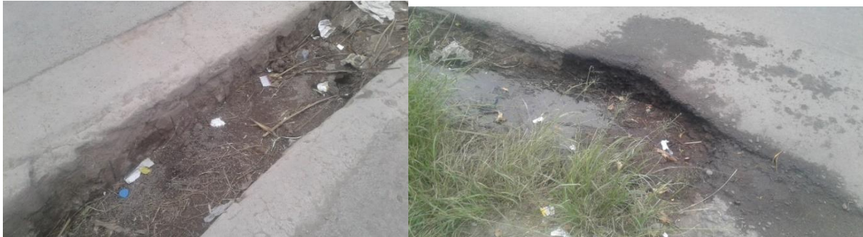
Figure 4-8: Lack of Frequent Clearance of Drainage system
