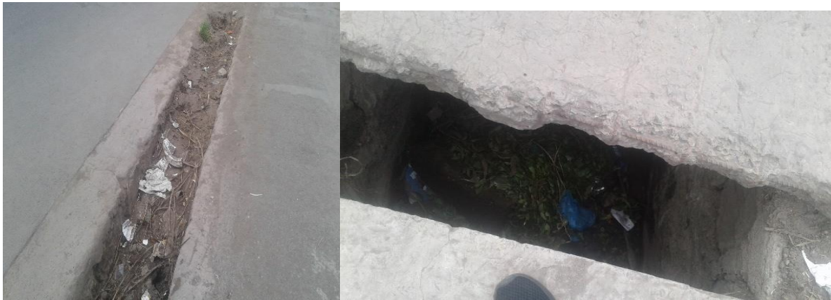
Figure 4-6: Dumping of solid and liquid wastes in to stormwater drainages
