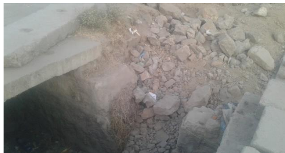
Figure 4-7: Damaged drain lines due to construction
