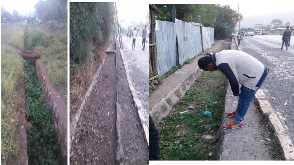
Figure 4-2 Drainage line filled by grass and sediment
