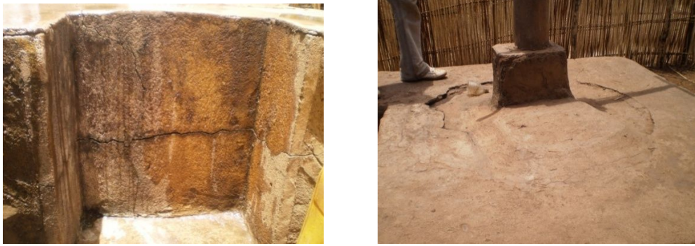
Figure 17: Cracks on head wall and top slab
