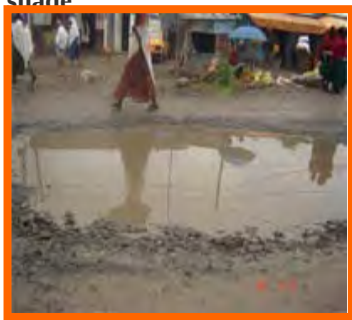
Fig.47. Deteriorated road Source:-Field Data, 2007
