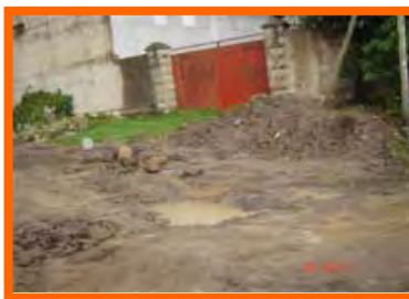
Fig.96. Photo showing deteriorated road.
