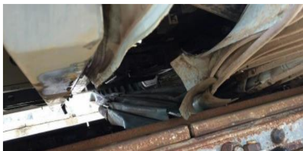
Figure 1.2: Damage to the gangway at AALRT.
