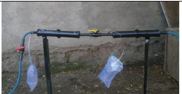
Moisture and hydrogen sulfide scrubber
