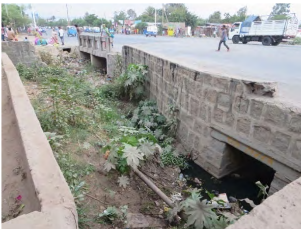
Photo 1: Existing slab culvert and the newly constructed box culvert (Right side of the road)
