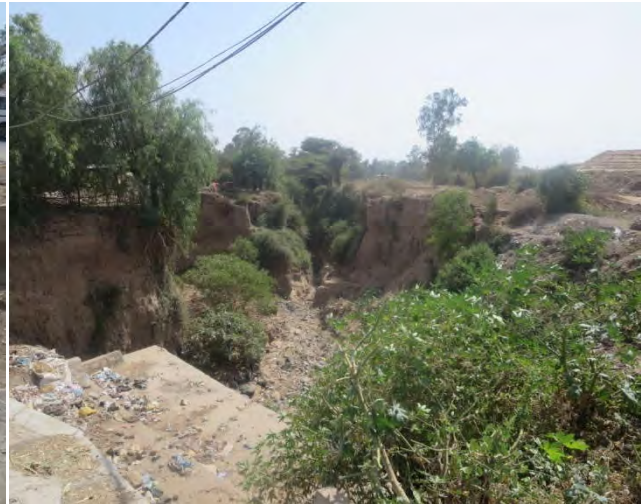
Photo 8: Eroded River bank at downstream side of the structure (Left)
