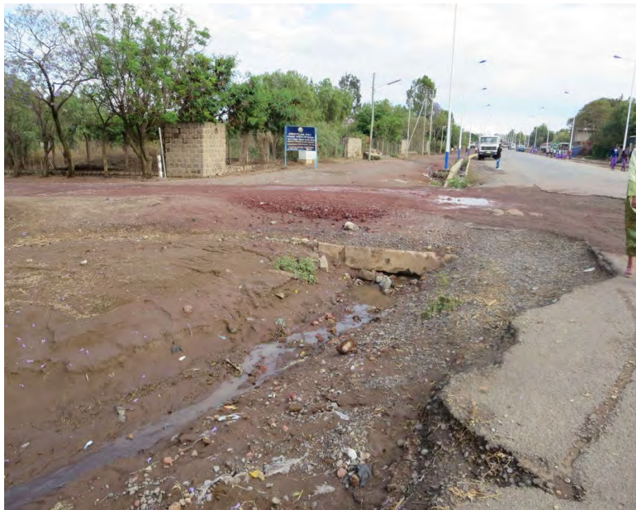
Photo 6: Overtopped and Damaged Asphalt Road Section around Km 3+300
