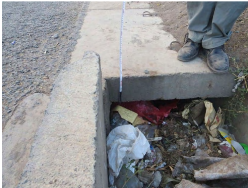
Photo 13: Side drain logged by dirt which has only 15cm water way.
