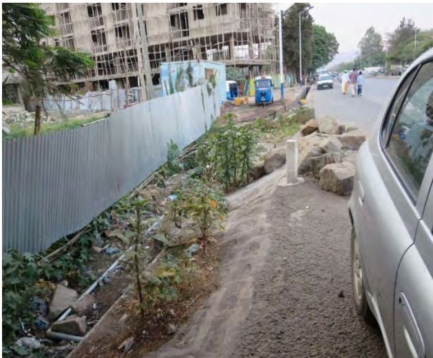
Start of the Project Road Photo 9: Side drain connection between Municipality & Nazerete-Assela Road Project (Right)
