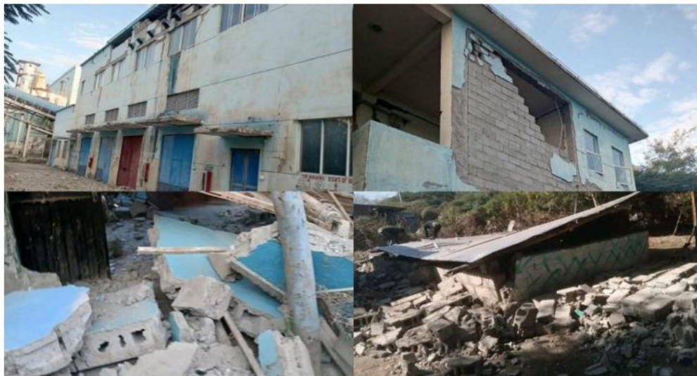
Damage to houses in the Afar area (image: Addis Standard)
