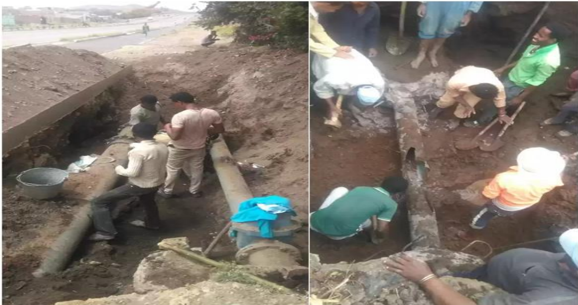
Figure 4. 4: Maintenance of Pipe Burst Observed During Field Visit.
