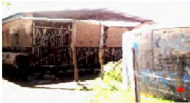
Fig 5.2: 40 m 3 Ferro cement reservoir fixed with a nearly damaged school block (Choki School)
