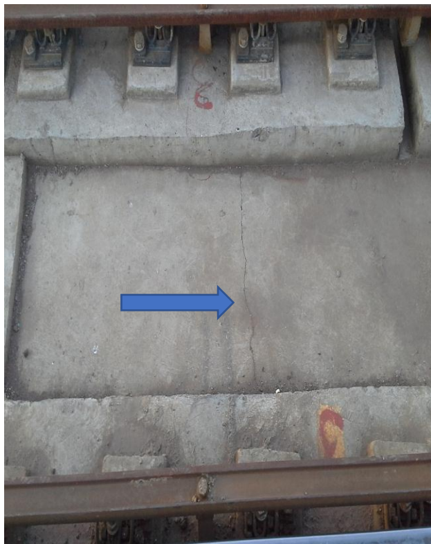
Fig. 3.6 Base Crack around Mexico station AALRT/Ethiopia
