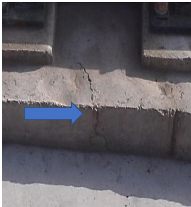
Fig. 3.4 Cracked Slab Track (Slab Sleeper) around Stadium station AALRT/Ethiopia
