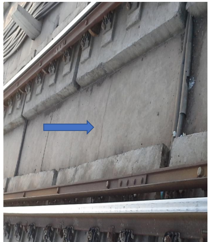
Fig. 3.7 Base Crack around Mexico station AALRT/Ethiopia
