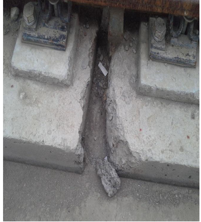
Fig.1.4 Crashed sleeper at Mexico station
