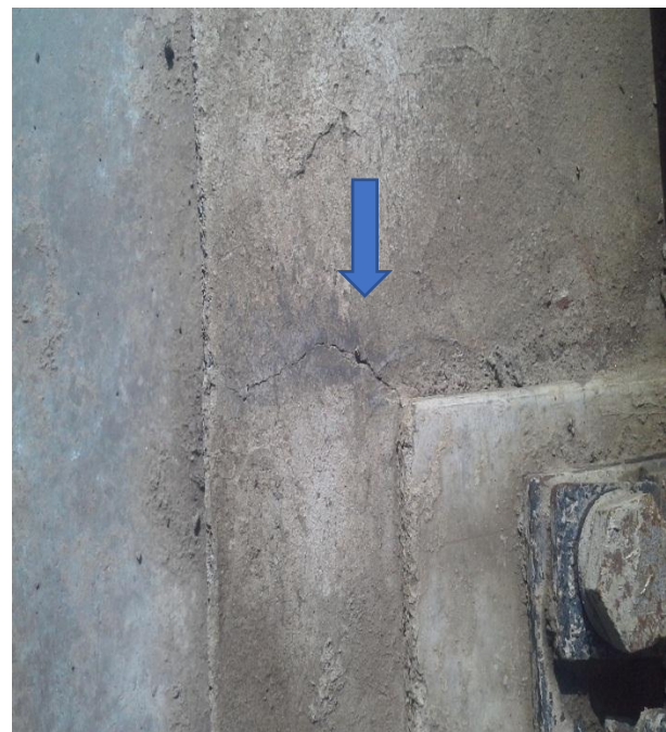
Fig. 3.5 Cracked Slab Track (slab sleeper) around Stadium station AALRT/Ethiopia
