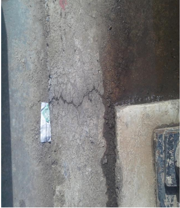
Fig.1.3 Cracked sleeper at stadium station
