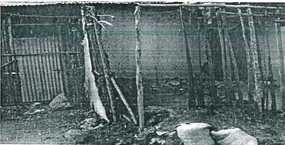
Figure 5.7 A partial view of demolished squatter houses and the bridge under construction
