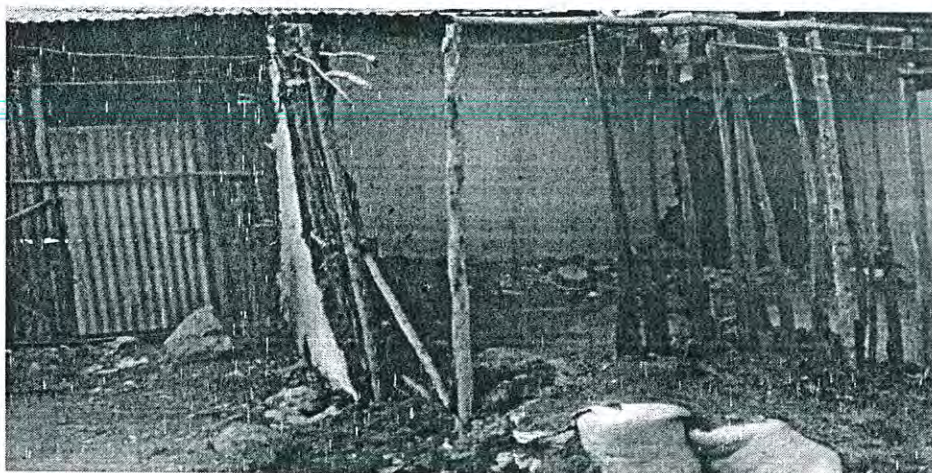
Figure 5.7 A partial view of demolished squatter houses and the bridge under construction
