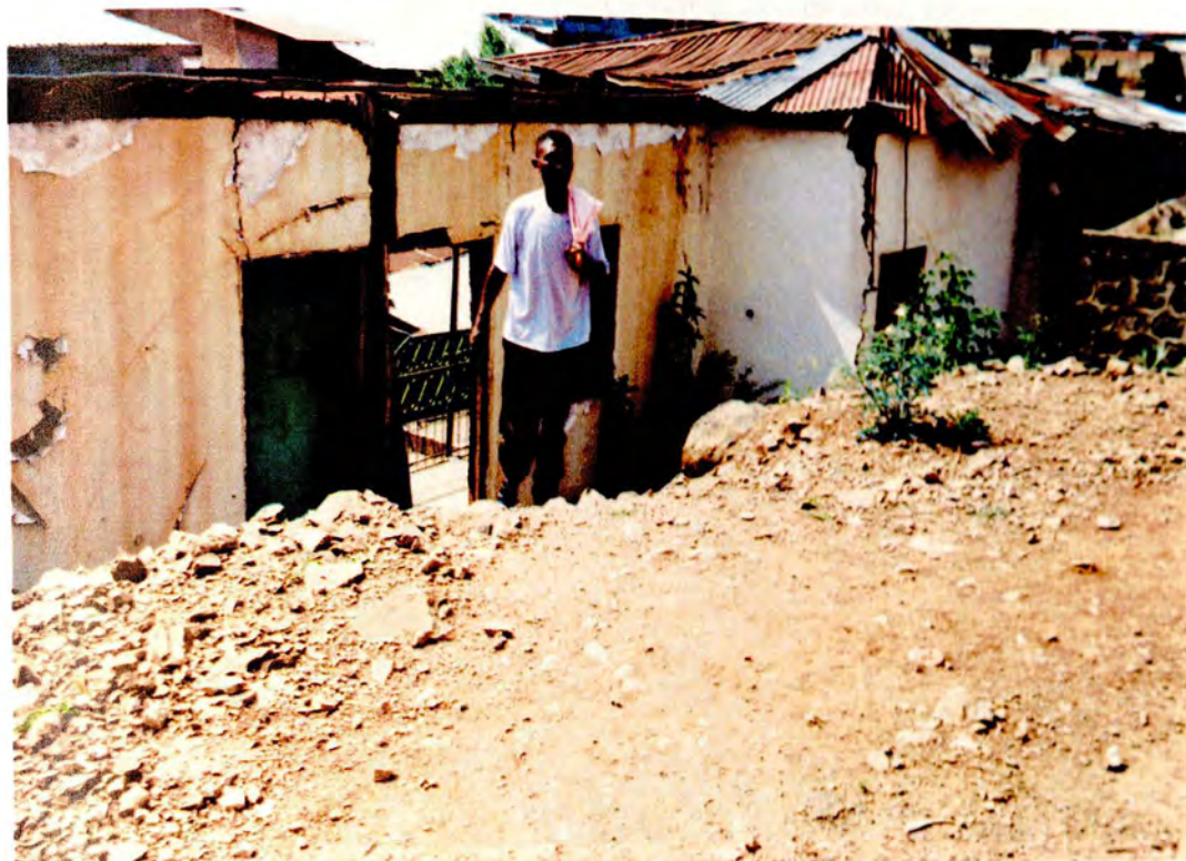
Plate 10: owner of partially demolished house in front of his house
