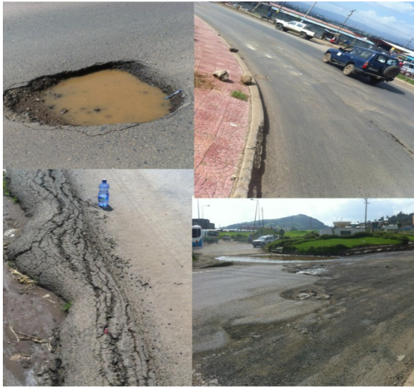
Plate 2.19 Pothole, Shoving, Rutting and Raveling distress types
