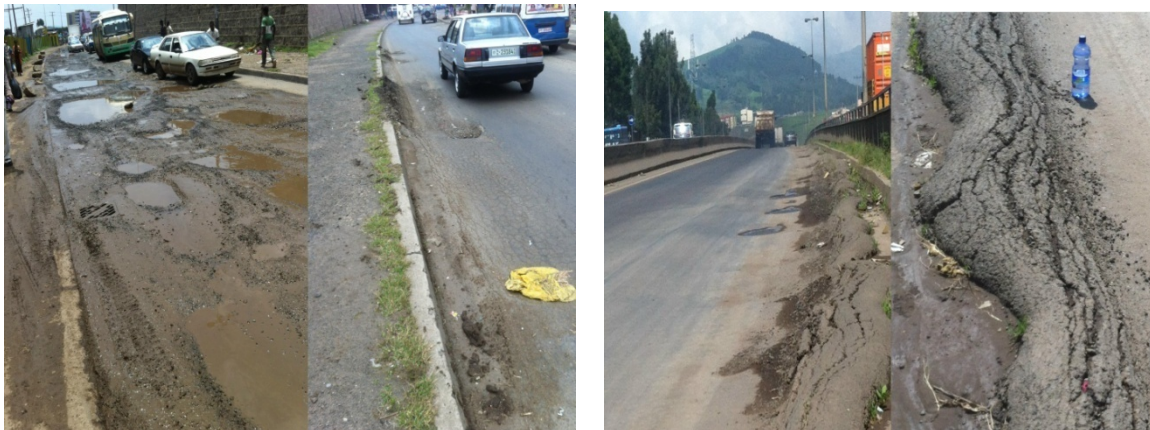
Plate 1.1 Pavement distress in the study area around Bole Brass and on way Kality to Hana Mariham, respectively
