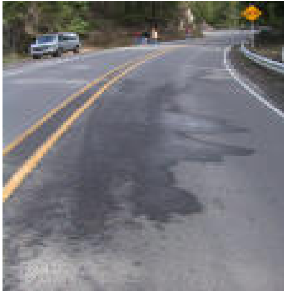
Plate 2.5 Bleeding on the road surface
