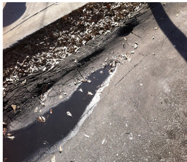
Plate 2.10 Rutting on the Wheel-path
