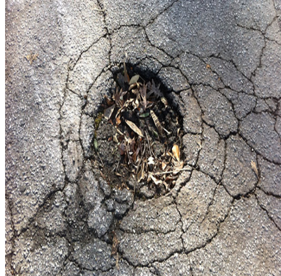
Plate 2.12 Potholes with alligator crack
