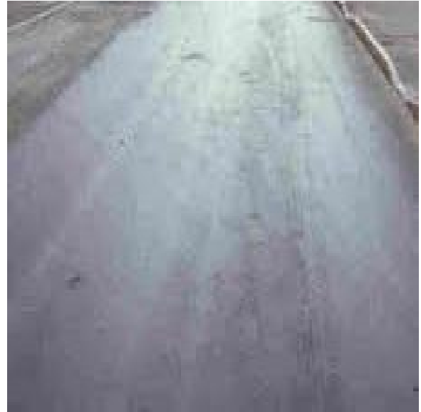
Plate 2.6 Fattening-up of the road surface
