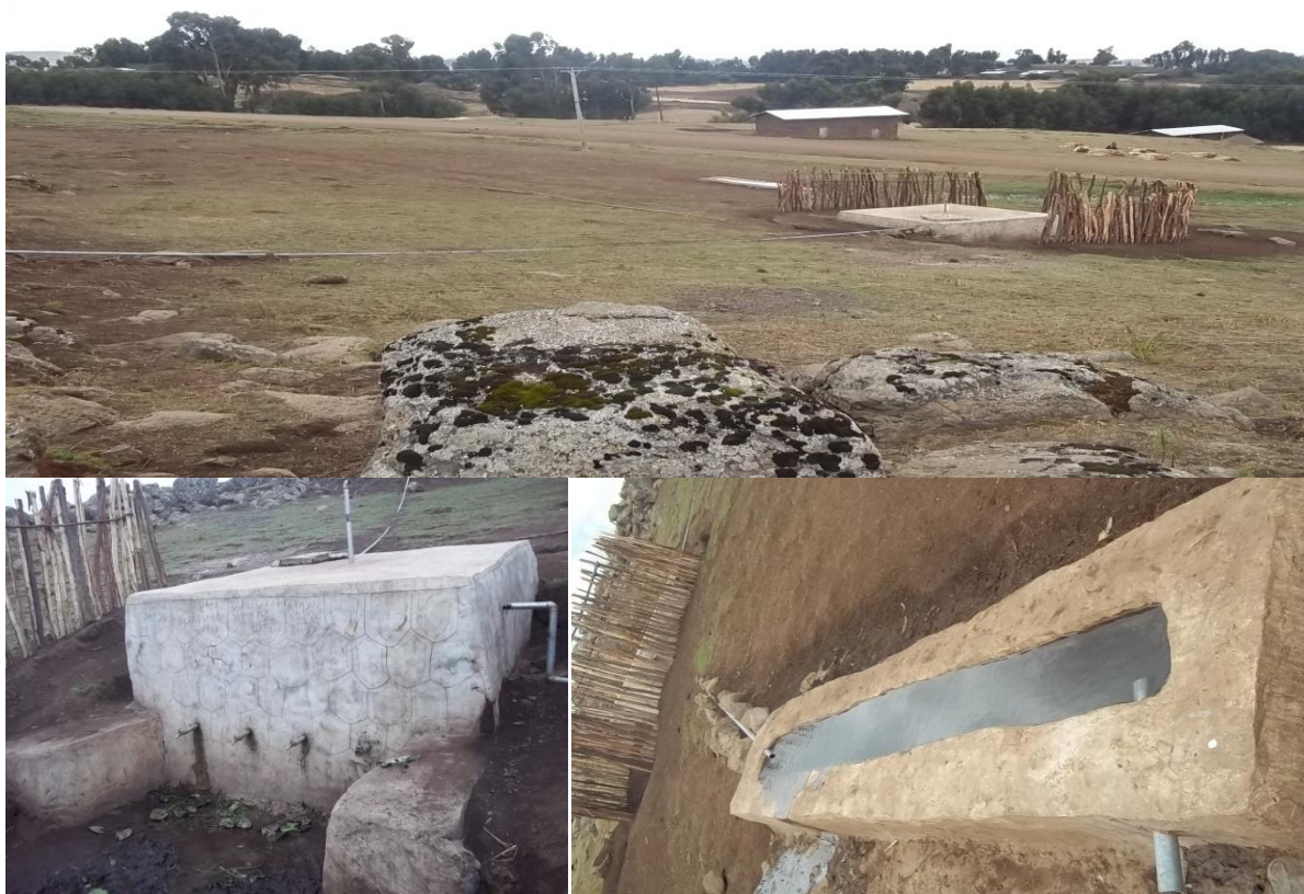
Plate 3: Mechanized highland stream water (Dangulé 15 February 2014)
