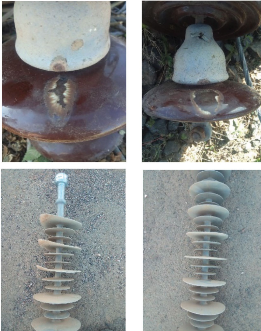
Figure 8. Examples of insulators damaged by pollution flashover events.
