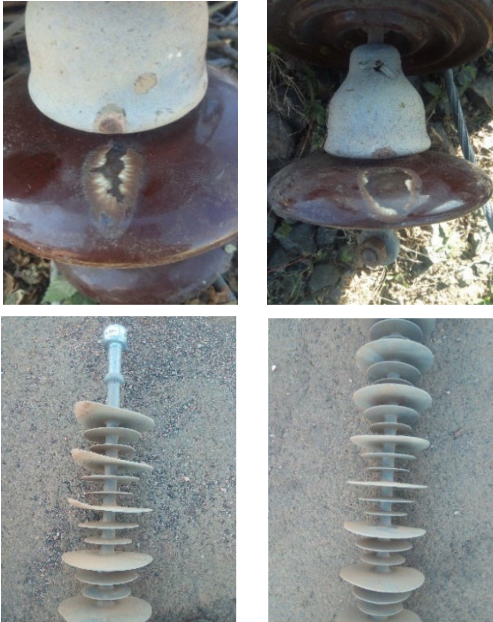
Figure 27: Examples of insulators damaged by pollution flashover events.
