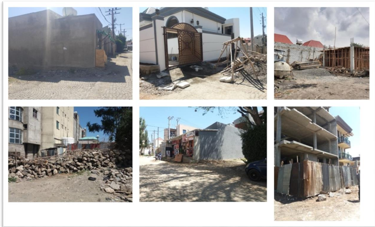
Figure 5: Green Area Violation at Lafto Micael
