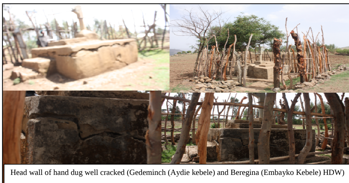
Figure 10: Cracked hand dug wells
