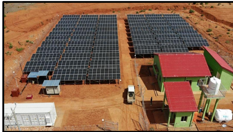
Figure 3.5 Qorile village 325kW solar mini-grid
