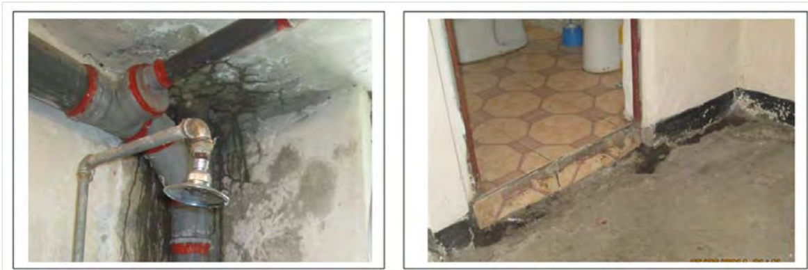
Figure 21: A sealed sewage line and leakages in one of the units of the condominium (pictures by author)
