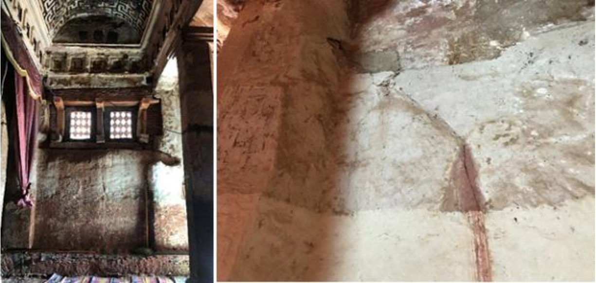
Figure 37: water leakage through the window and crack.
