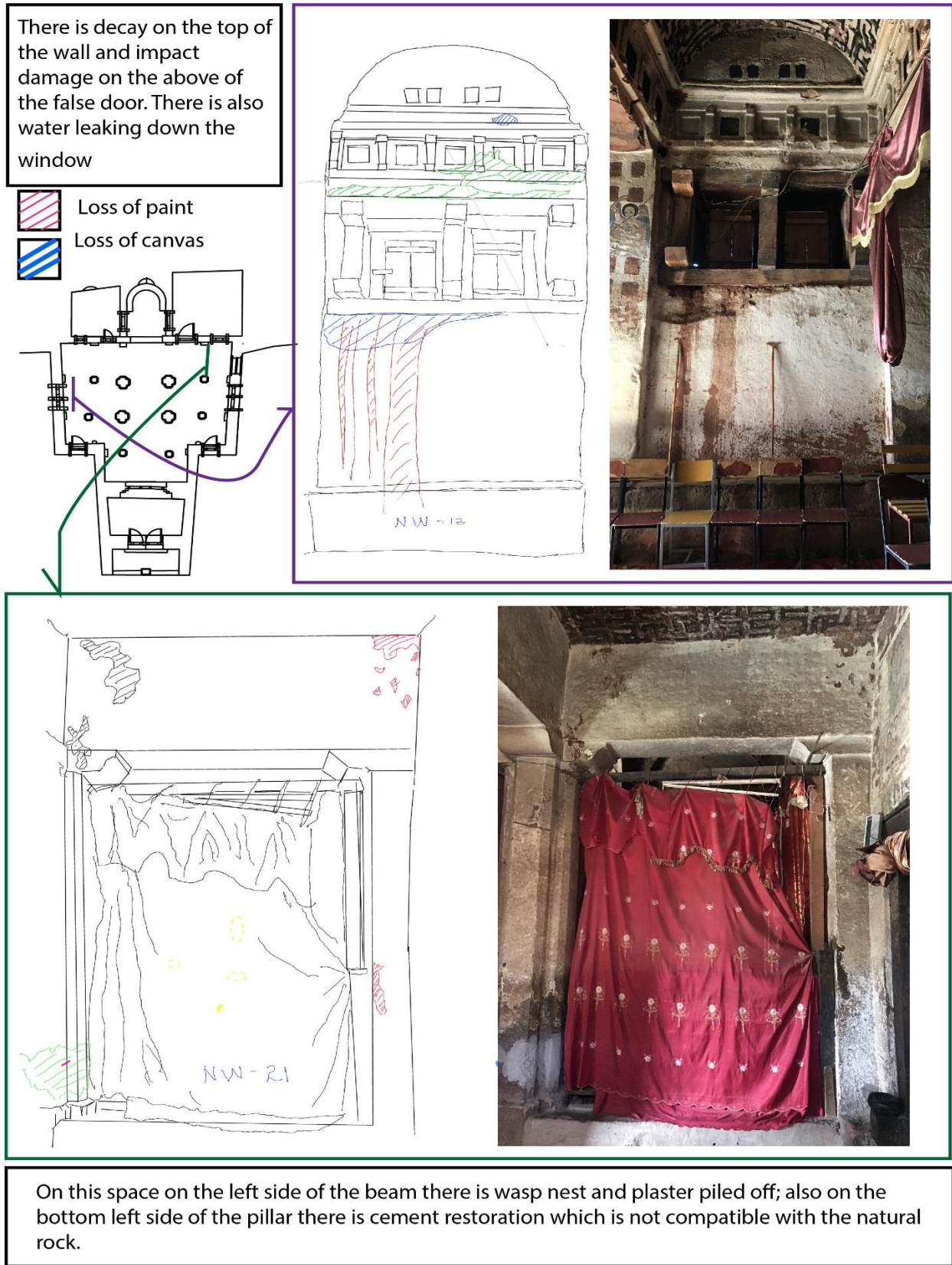
Figure 54: deterioration analyses of the wall at the Qidest.
