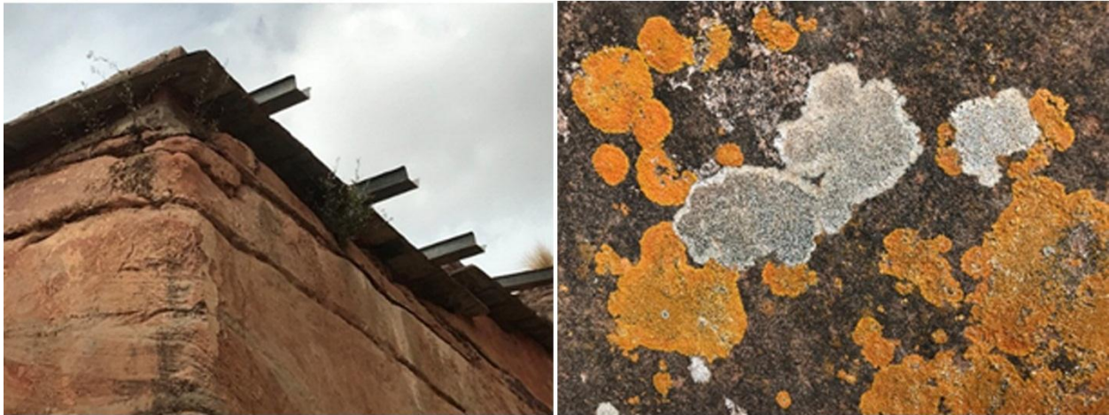
Figure 36: lichen and plant growth.
