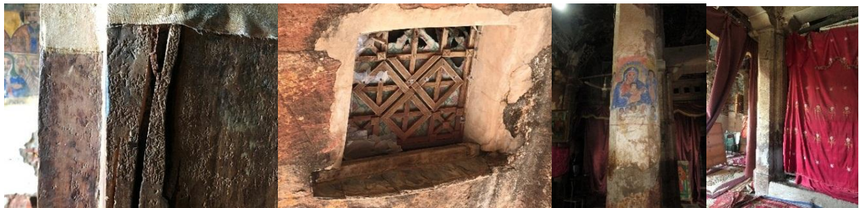
Figure 38: poor conservation practice.
