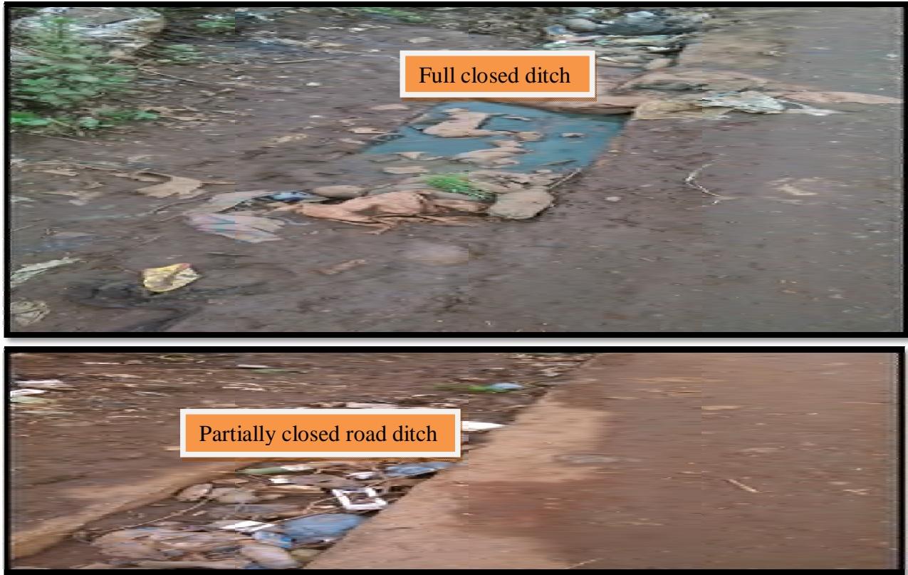
Figure 2.2: Typical silt loaded ditch
