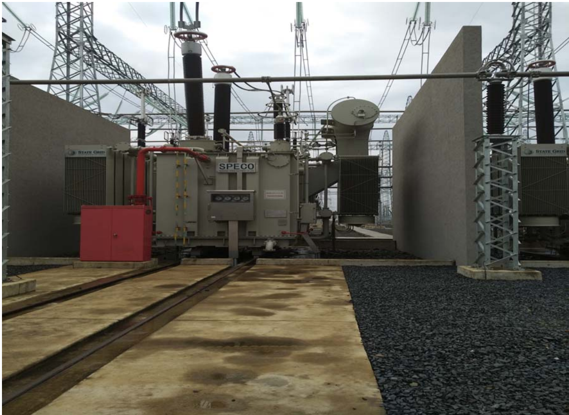
Figure 3.2: Single phase 500/400 kV autotransformer.
