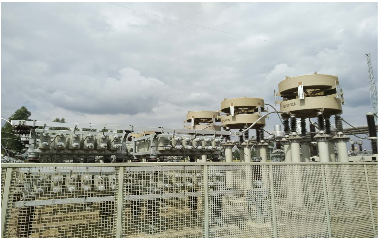
Figure 1.5: TCR and TSC equipment at HOLETA 500/400 kV switchyard
