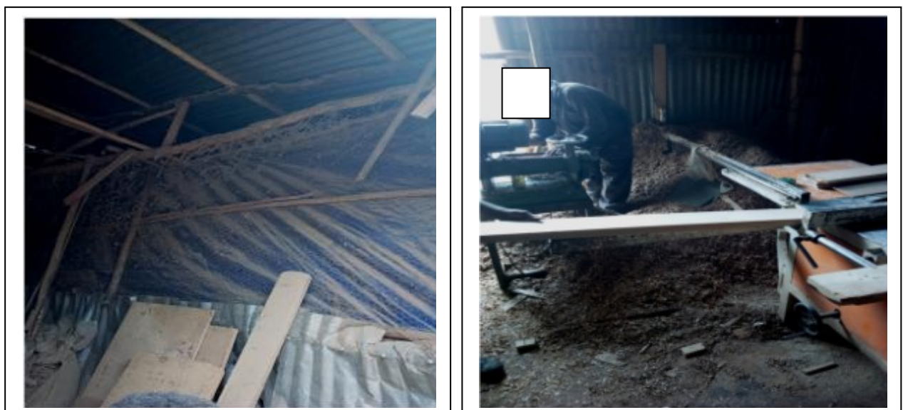
Figure 10: Dust accumulation on the wall (Photograph by Tegegnetwork Yitayew)
