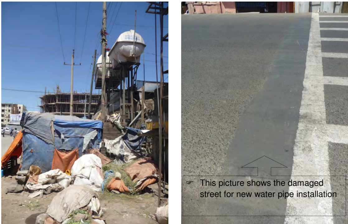
Figure 2.9: Shows crowded electric poles and damaged paved street respectively
