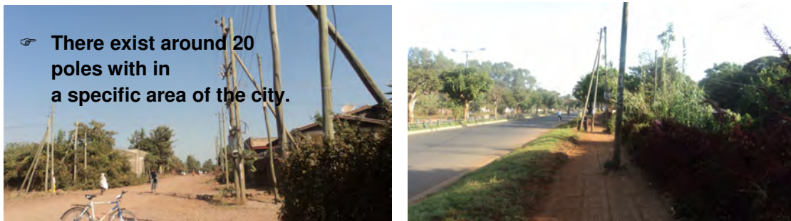
Figure 4.9: Both figure shows improperly located electric poles
