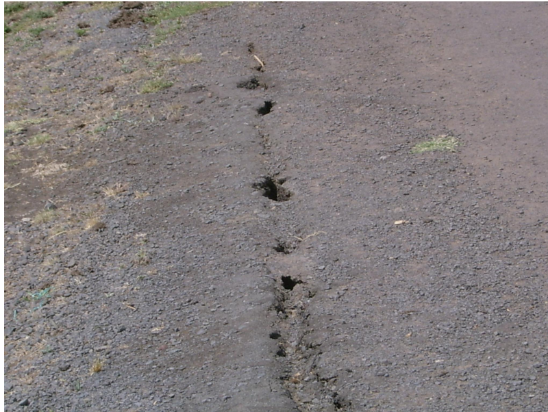
Plate 6-3 Longitudinal cracking along left side of the road (km32+150)
