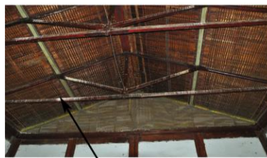
Internal parts of the hall ceiling damaged due to bird droppings
