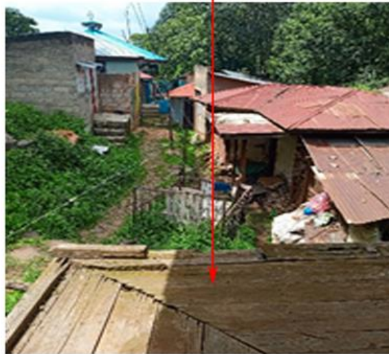
Deteriorated and damaged floor due to rain
