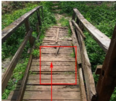
Deteriorated floor of the ramp due to rain and age
