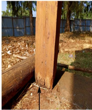
Damaged by rising damp
