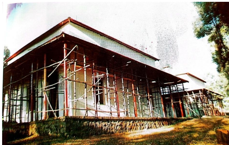
Figure 19 The damaged Palace Building during renovation,1999
