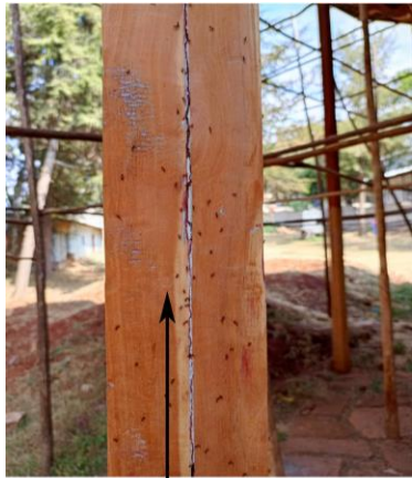
Damaged by insect
