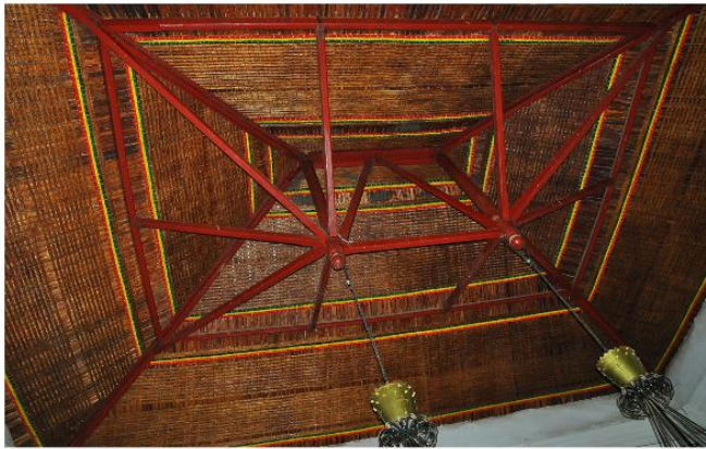
The Beam serving as a ceiling and structural bearing at the external corridor parts
