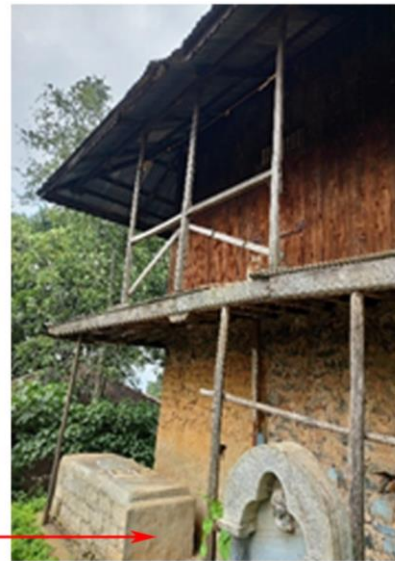
Figure 65 Current condition of floor in Nebir'ed residence
