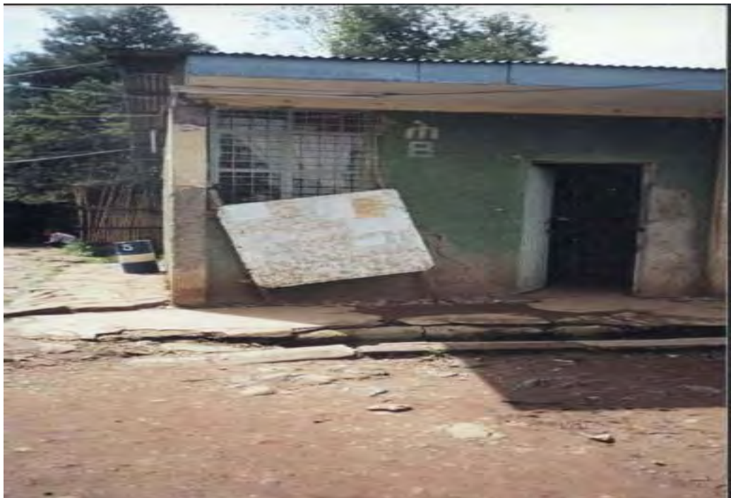
Figure 2.3.1 Detachment of Tie beam and column in Bole senior secondary school [3]
