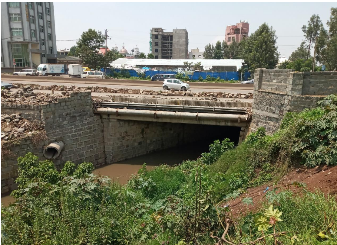
Figure 5.6 Scattered brush and heavy weeds along river channel
