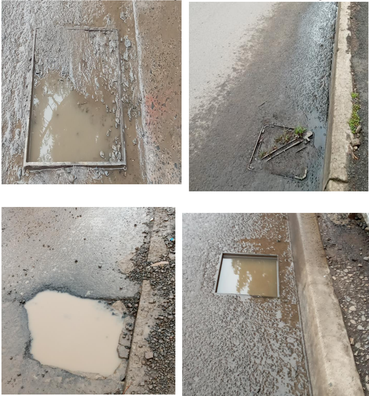
Figure 5.11 Damaged inlets and inlets clogged by rubbish
