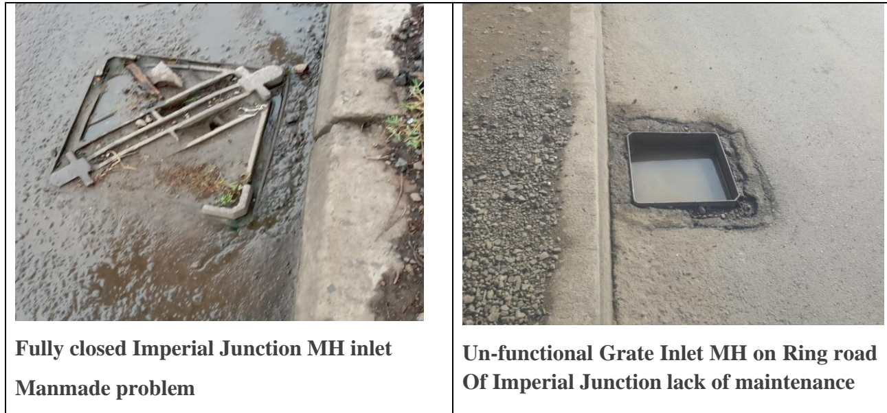
Figure 3.2 storm Drainage along the ring road
