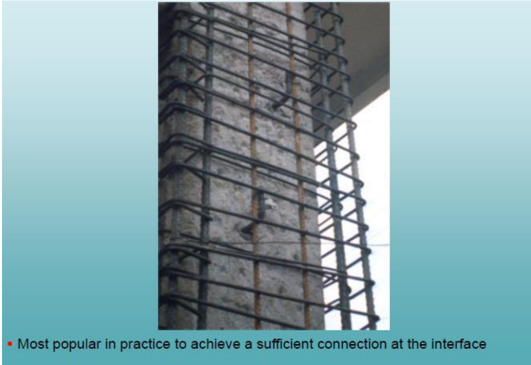
Figure 15: Use of steel dowels and roughening the surface of an original column to achieve connection at the interface
