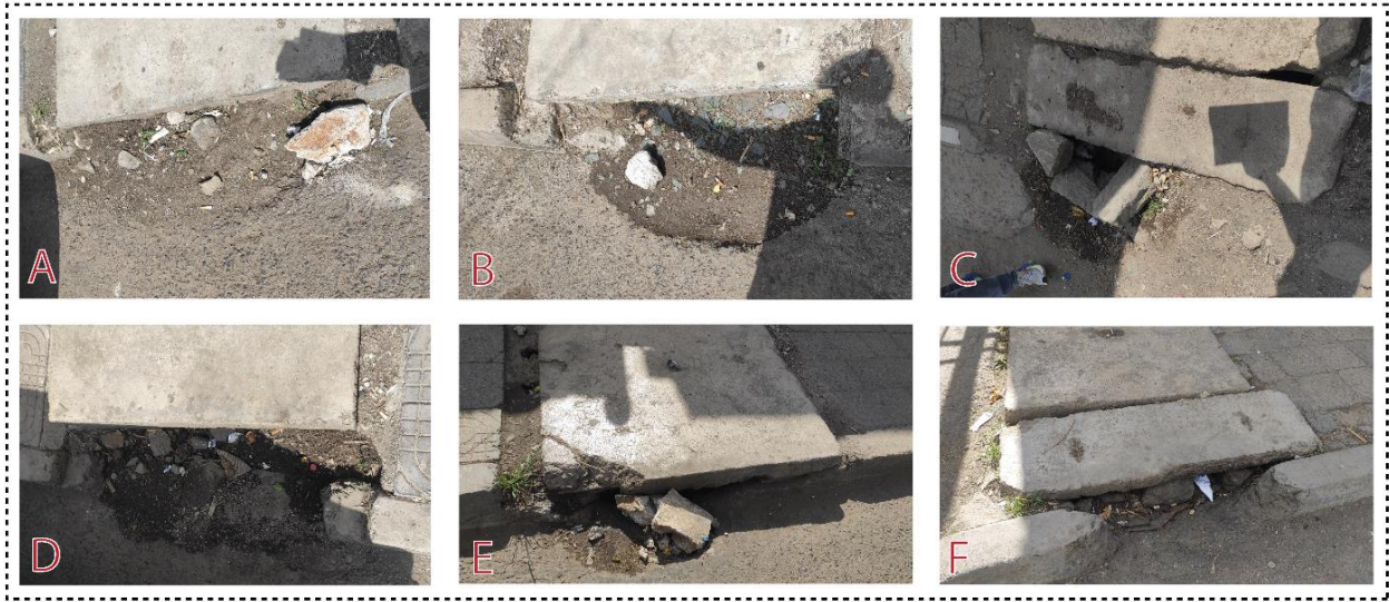
Figure 4.15: Stormwater Drainage conditions (9.0119552, 38.819920)
