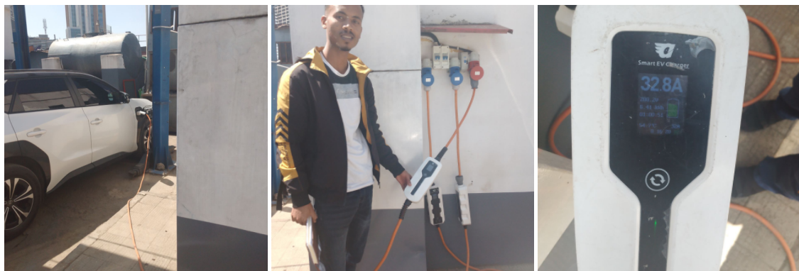
Figure 3.7: Electric Vehicle Charging Station at Meskel Flower Stadium
