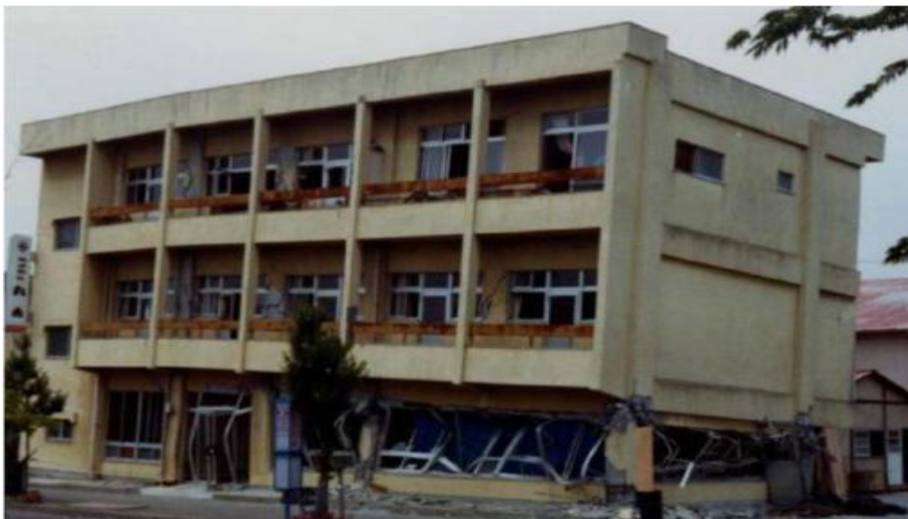
Figure 2.9: Damage from irregularity during 1978 Miyagi – Ken – Oki Japan earthquake (Ellingwood 1980):
