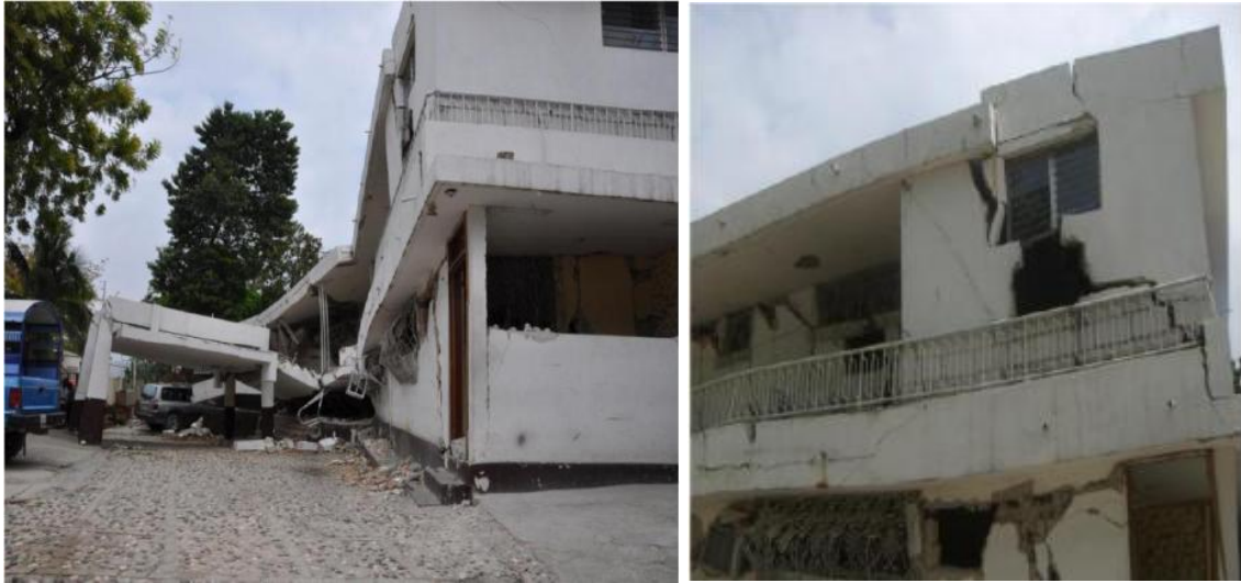
Figure 3.0: Damage from Irregularity during 2010 Haiti earthquake (Mid America Earthquake Engineering Center, University of Illinois at Urbana Champaign)
