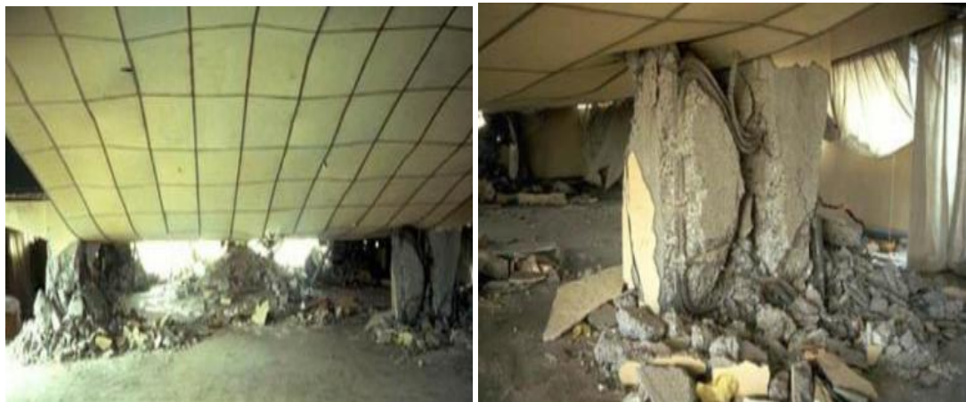
Figure 2.8: Damage due to irregularity during Guatemala earthquake 1976; Collapse of second storey due to shear failure of column
