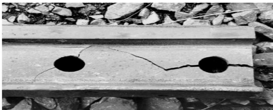
Figure2.6: Web cracks originating from a fishbolt hole [16].
