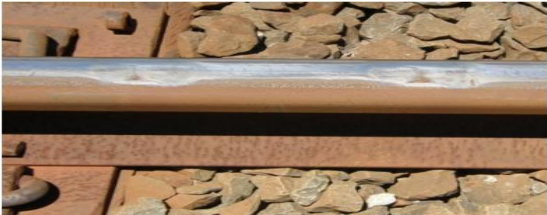
Figure 2.2 :Squat: damage of the running surface (“hot spot” and crack nucleation) [8].
